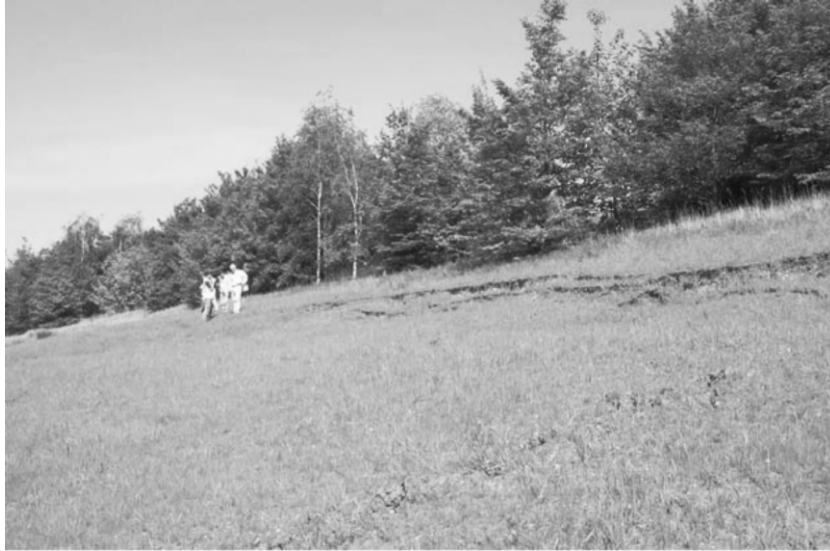
Figure 3. Instability of cutting slopes on the M11 near Loughton. Adjacent vegetated areas appear more stable.
