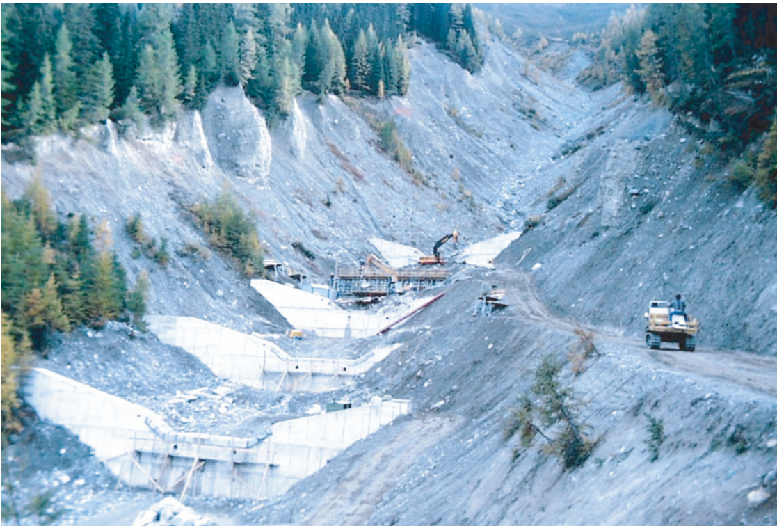
Figure 7. Middle reach of a torrent with deeply eroded moraine deposits. Technical countermeasures (concrete consolidation dams) were under construction in 1991.
