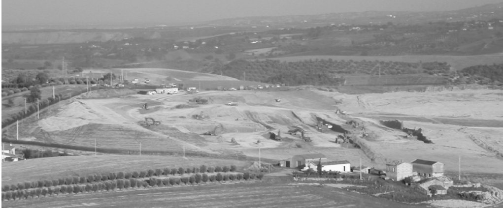
Figure 2. Excavation of the hills for the preparation of the site where the power station is under construction.
