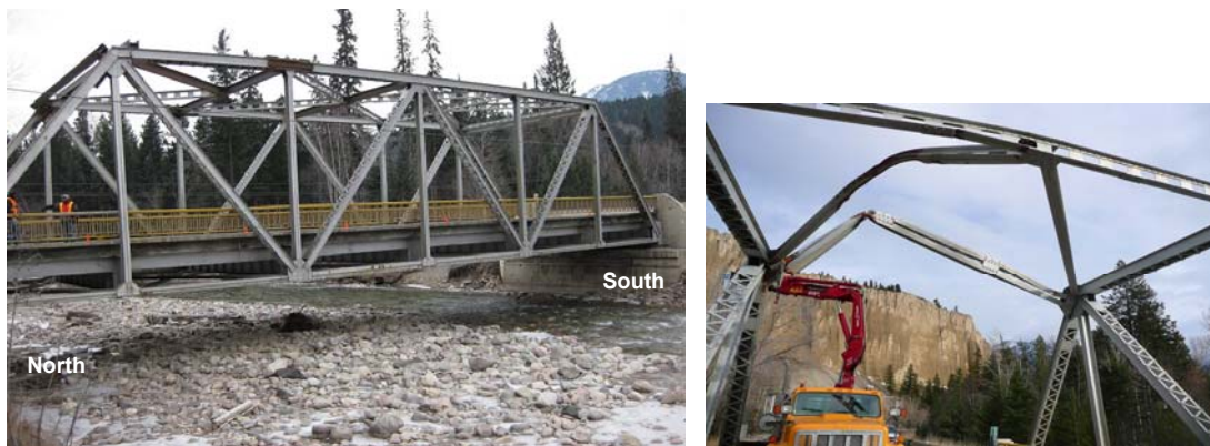
Figure 3 Overall view of Dutch bridge and damage to the truss
