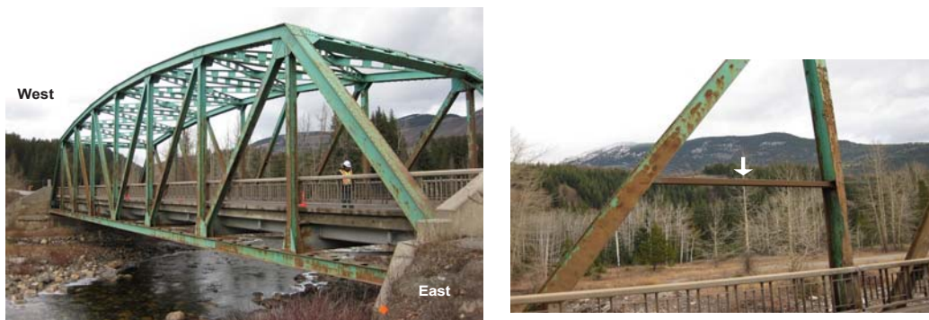
Figure 4 Overall view of Loop bridge and partial repair to damaged truss
