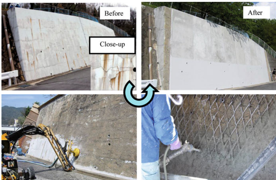
Fig. 7.7 Surface repair of retaining wall. Counter-clockwise: appearance before rehabilitation, surface preparation with high-pressure water-jet, application of SHCC, after rehabilitation (Rokugo, 2005).
