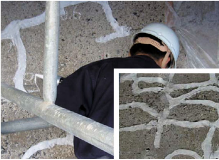
Fig. 7.6 Existing cracks are being sealed with a polyurethane sealant to prevent bonding with the SHCC and the substrate over a width of 30 mm (Rokugo et al., 2005b).
