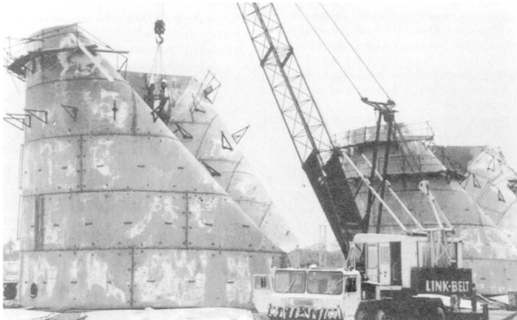
Figure 1.1 Collapsed oil tanks in West Africa (2 of 6 similarly damaged tanks shown): After Schaden Spiegel 2/94 1,3
