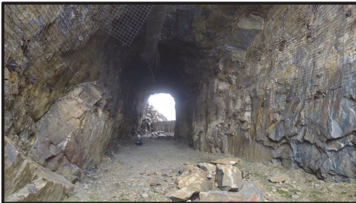
Photograph 3. Looking southwest with both rock falls visible; note angled tunnel walls
