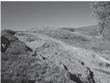
Photograph 5. Erosion in Service Spillway
