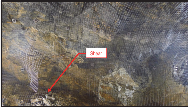
Photograph 2. Failed mesh and loose rock in mesh near tunnel middle; partial source of rock fall
