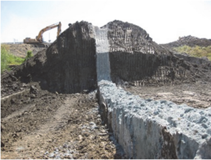
Photograph 2. East Levee over-excitation of CB cutoff wall at pump station outfall.
