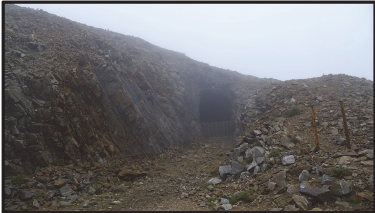
Photograph 1. Southwest portal overview; note loose rock on left side and low cover over tunnel
