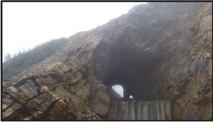
Photograph 4. Northeast portal overview looking southwest; note the low cover over the tunnel
