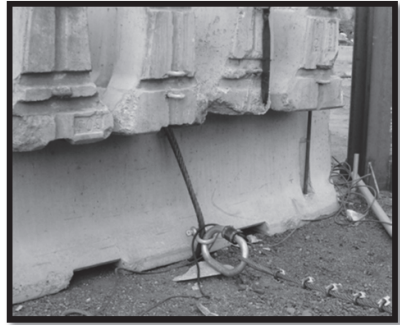
Photograph 11. Link cell of uphill wire rope anchors attached to the concrete barrier system.
