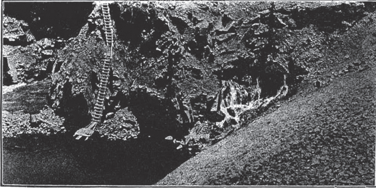
C. SOUTH MARGIN OF THE DAM ON THE DOWNSTREAM SIDE, SHOWING LEAKAGE AROUND THE SOUTH END OF THE DAM.
