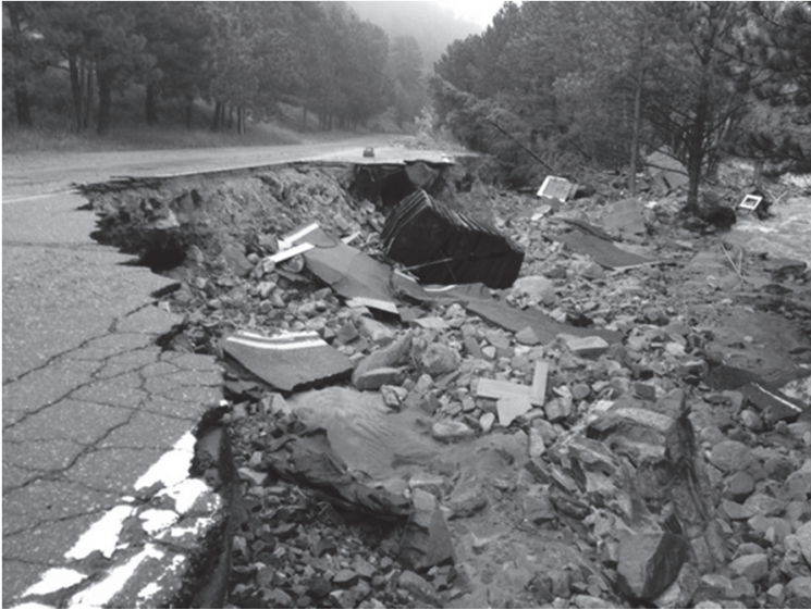
Photograph 1. Damage along James Creek
