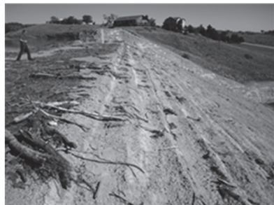
Photograph 6. Damage in Emergency Spillway
