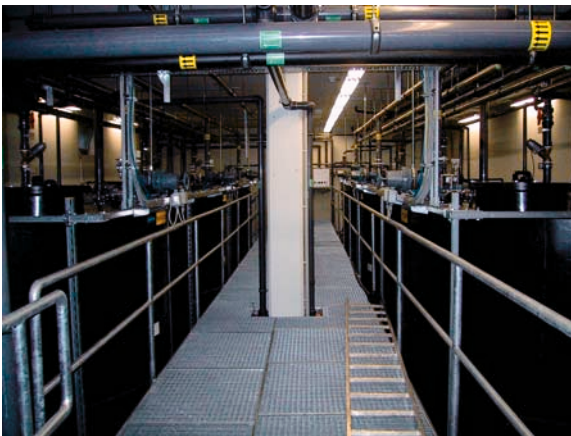
Fig. 22.3. Waste disposal area at the Department of Nuclear Medicine and Endocrinology, PET/CT Center Klagenfurt
