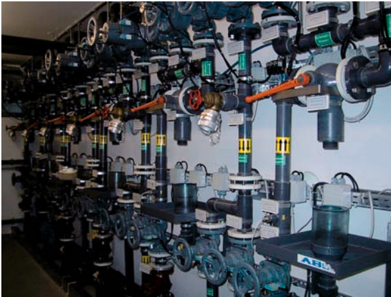
Fig. 22.2. Waste disposal area at the Department of Nuclear Medicine and Endocrinology, PET/CT Center Klagenfurt
