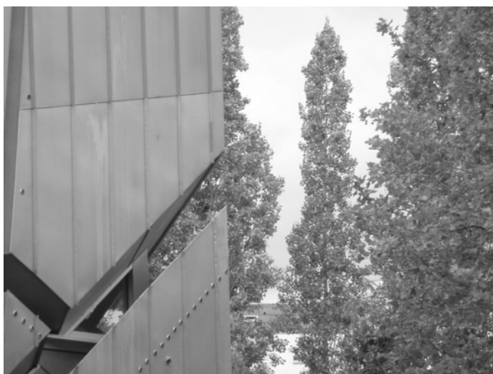
Figure 8-4. Exterior, detail view of exterior wall with opening. Photographed by Frank H. Weiner.
