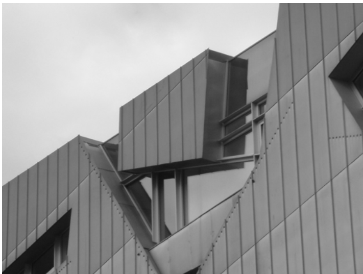
Figure 8-3. Exterior, detail view of wall with parapet and windows. Photographed by Frank H. Weiner
