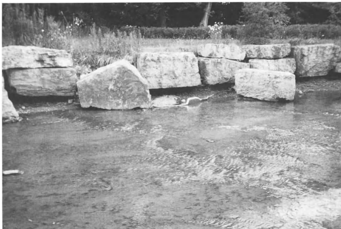
Figure 4. Undercut (45 cm), and toppled armour stone bank protection at Atwater Reach. Flow right to left. MAF flow depth is just over the armour stone, about 1.6 m. The stone on the right traveled 43 m to its present position (from site mapped in Figure 8) during the Opal event. Notice the flat bed to the stream rising only slightly at the channel margins under the blocks.
