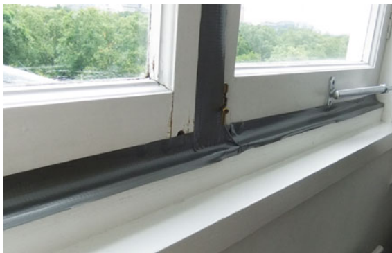
Fig. 14.4 A taped window to reduce air infiltration
