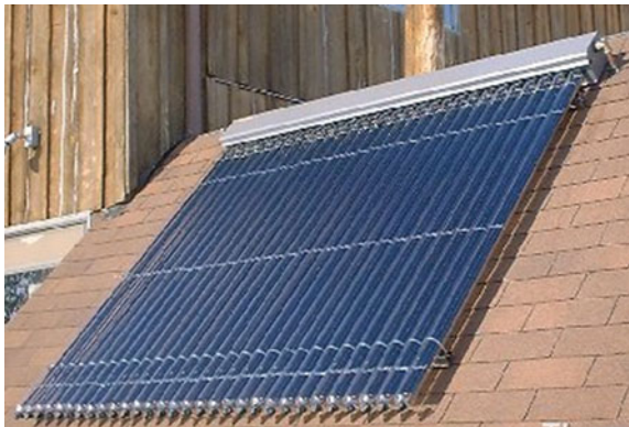
Fig. 11.6 Evacuated tube collector on a domestic tiled roof
