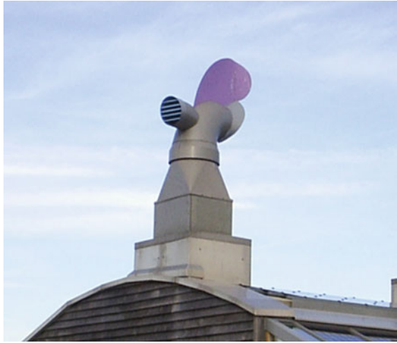
Fig. 10.8 Rooftop wind cowls (Image: Runming Yao)
