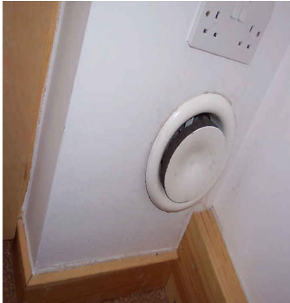
Fig. 10.9 Indoor air outlet fixed in the kitchen (Image: Runming Yao)
