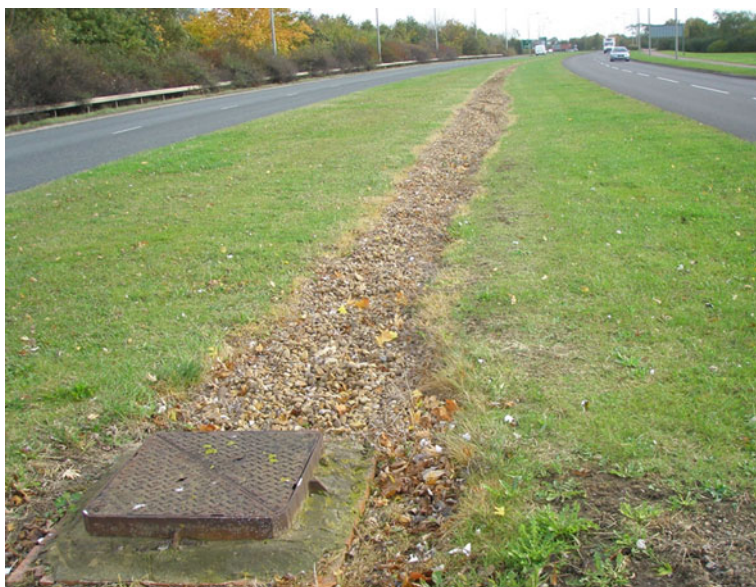
Fig. 7.8 An infiltration trench at a main road in Caldecotte, Milton Keynes
