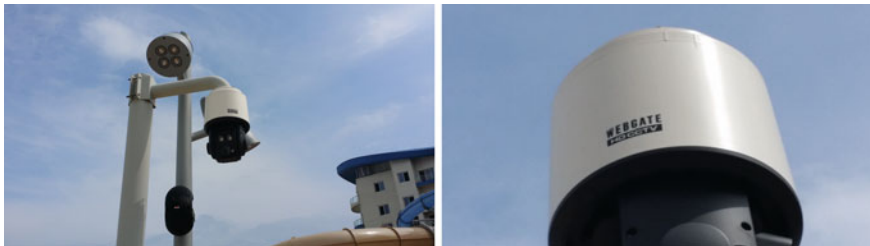
Fig. 1.37 Installment of CCTV cameras for safety and surveillance information in the aqua-world, Sol Beach Samchok, Gangwon province, Korea
