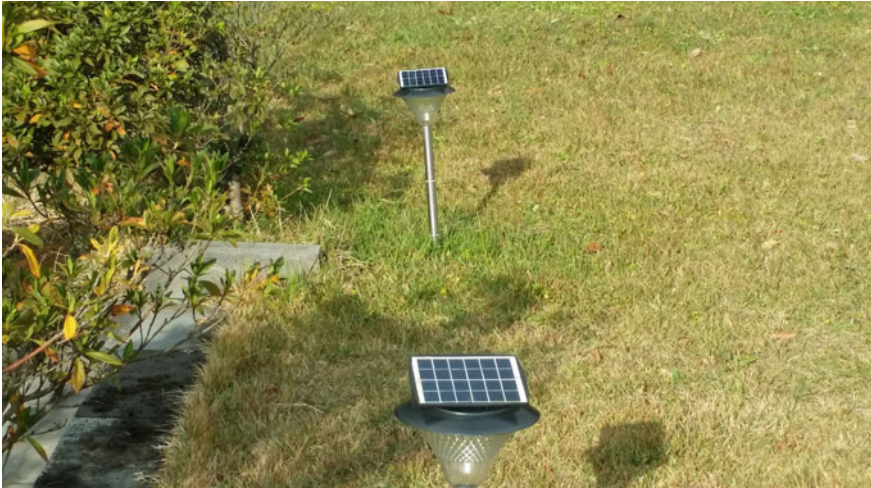
Fig. 6.12 Solar LED garden lighting, Jeju Island, Korea
