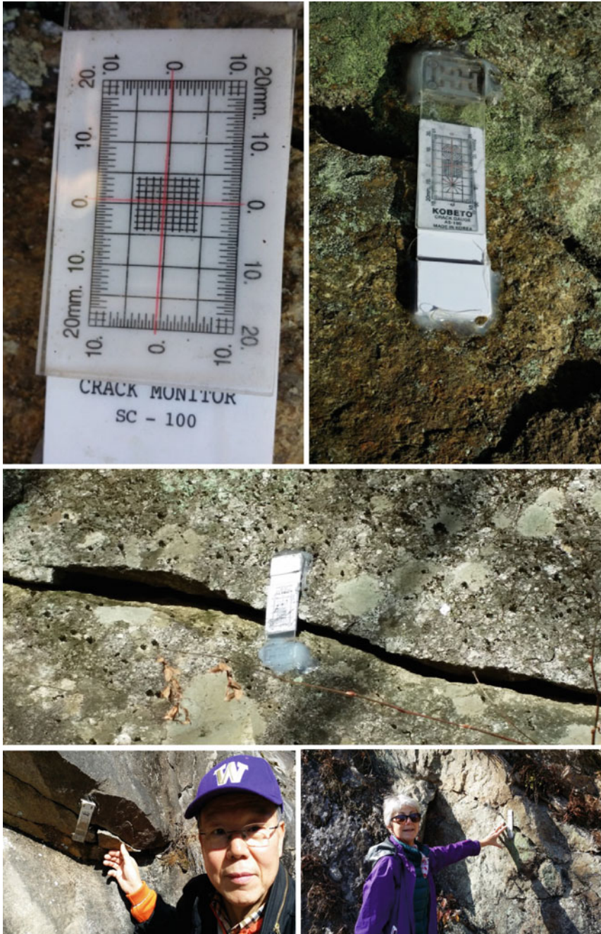
Fig. 4.31 Crack gauge to monitor horizontal and vertical movement across cracks on different rock surfaces, Seoraksan National Park, Korea
