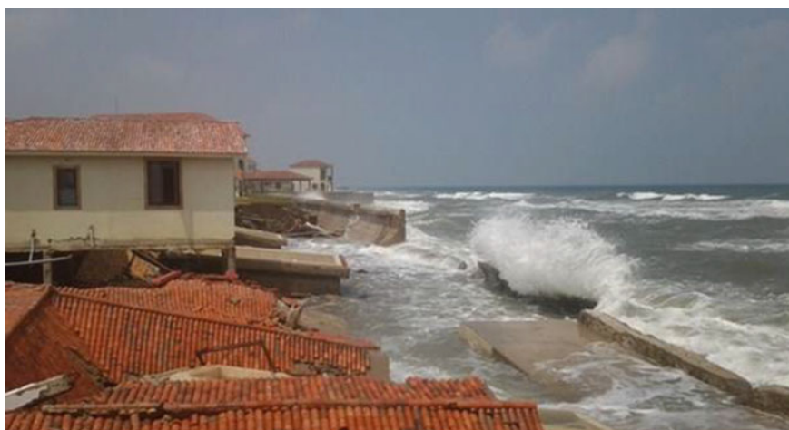
Fig. 4.10 Destruction of sea wall, Hoi An City, Vietnam
