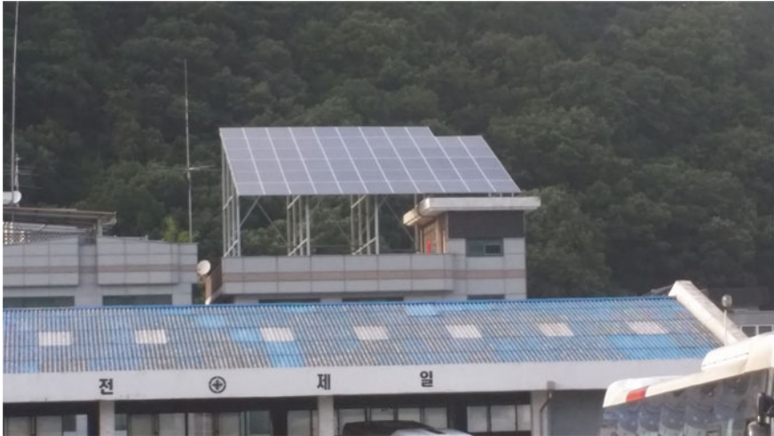
Fig. 3.5 Photovoltaic module, Hongcheon, Korea
