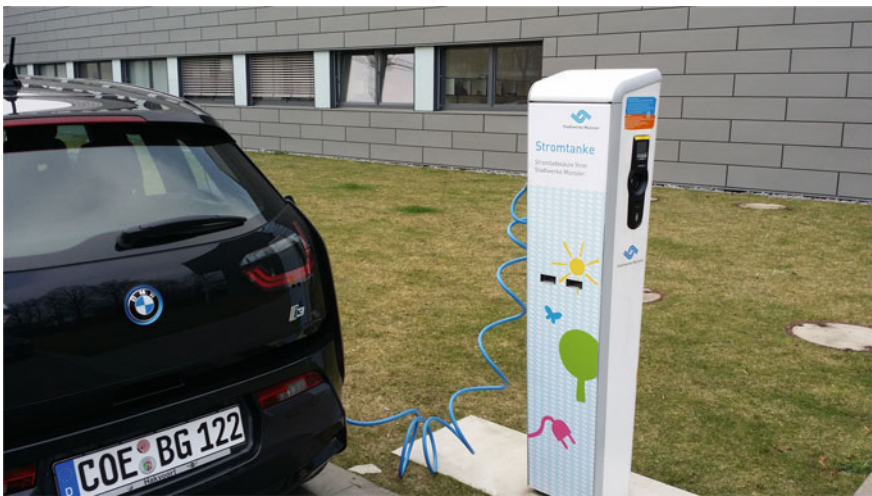
Fig. 3.4 Electric vehicle (EV) charger (charging station), Munster Electrochemical Energy Technology (MEET), Munster, Germany
