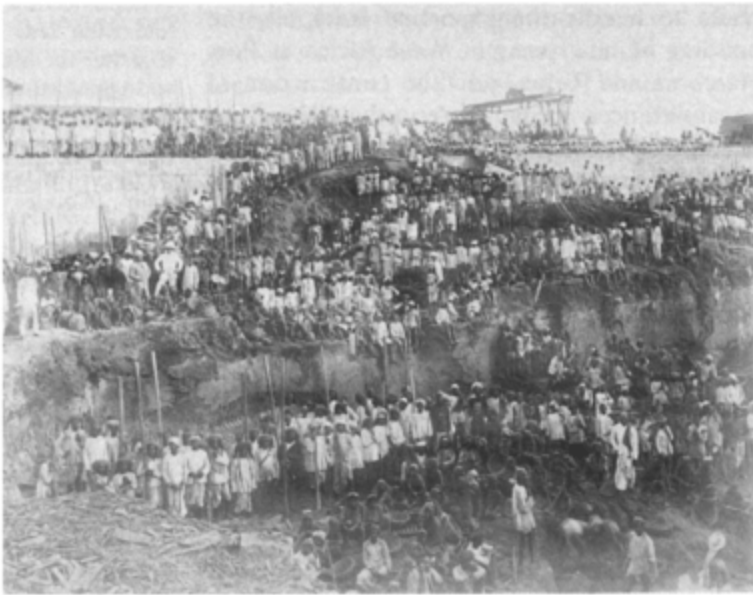
Prince's Dock. Extension work to the port of Bombay in 1887. These pictures, taken by the Port Trust, show the labour-intensive methods for large-scale excavation, and the drainage difficulties encountered. (Source: India Office Library)
