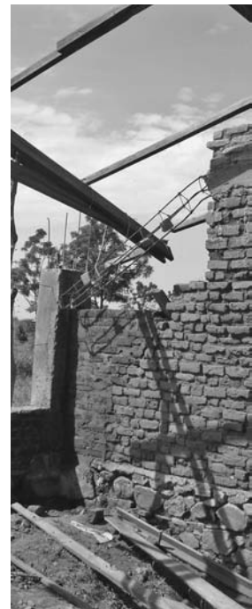
9.3 Crumbled church wall in Nyambogo, Tanzania. Photograph from Village Life Outreach.
