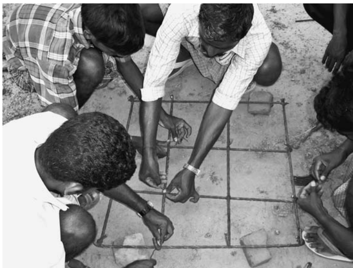
11.1 ARTES mason training program in [re]bar bending. Photograph by Durganand Balsavar in Nagapatinam district during the ARTES tsunami rehabilitation project, 2005.
