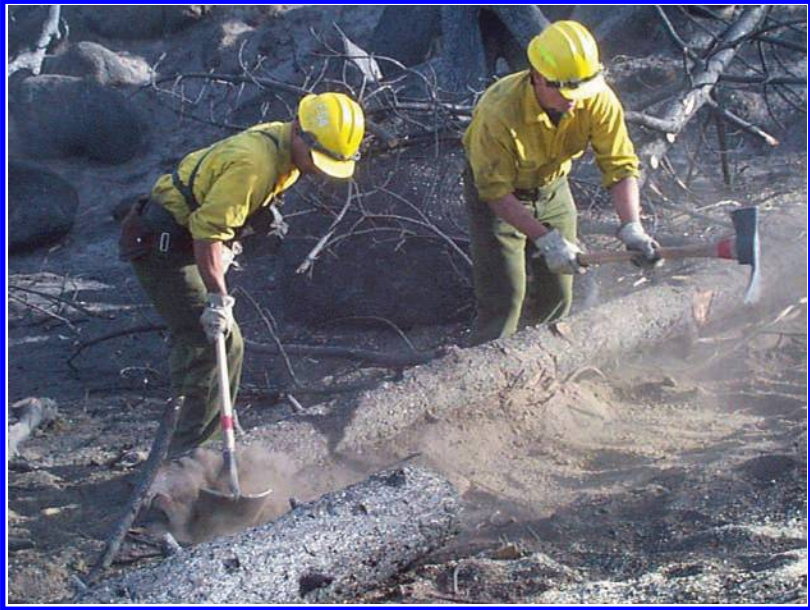
Fig. 5 Workers are digging the sediment storage basin upslope of a newly installation contour-felled log erosion barrier.
