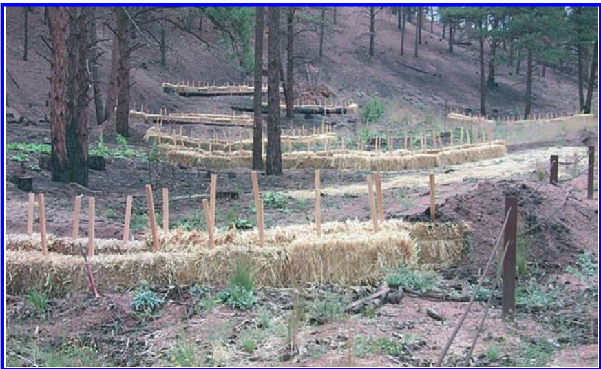
Fig. 4 Straw bale check dams were installed in a small swale below a steep slope after the 2002 Hayman Fire in Colorado, USA.
