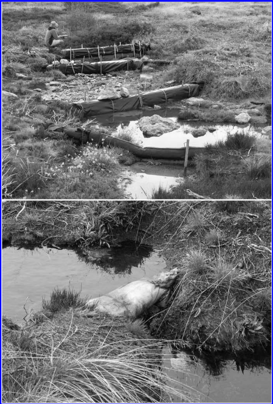
Fig. 5 Post-fire rehabilitation works on the Bogong High Plains, Victoria. Upper: a series of weirs constructed along an eroding drainage line. Lower: a weir retaining water in a burned area of moss beds.
