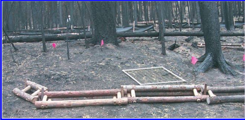
Fig. 4 Multi-log structure constructed for use as an erosion barrier. Effectiveness of this treatment is currently being measured using silt fence plots.
