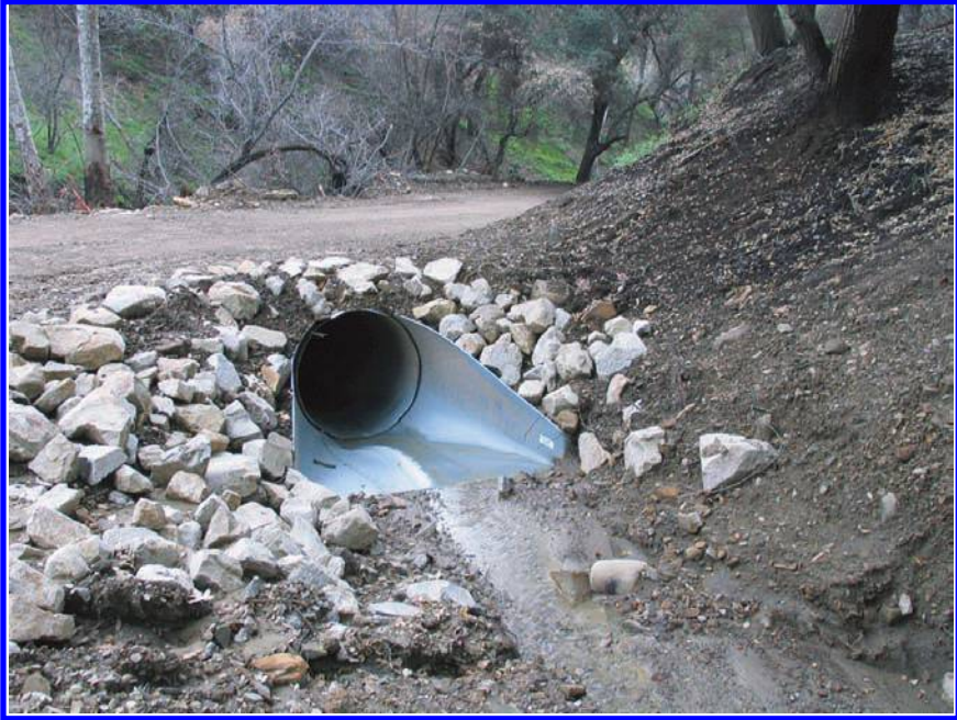
Fig. 3 A new, larger culvert and inlet armoring installed after the 2003 Piru Fire in southern California, USA.
