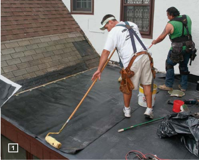
BRIDGE TRANSITIONS IN ROOF SLOPE. This transition between the house's low- and steep-slope roofing created ice dams that rotted a section of sheathing. In response, the author covered the transition with the EPDM membrane. Replacement shingles will be installed later.
