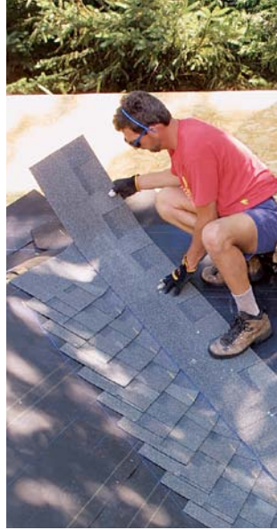
A ROW OF SHINGLES CREATES THE VALLEY. For a no-cut valley, a row of shingles is bedded in roof cement (left) and installed with their top edge on what would be the cutline (right).
