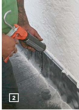
CAULK THE TERMINATION BAR. Urethane sealant fills the kick and coats the fastener heads.
