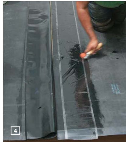
ROLL THE SEAM. The seam tape is rolled with a 3-in. neoprene roller.
