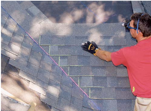
NO GUIDE LINE NEEDED. Shingles go in with one corner butted to the valley shingle.
