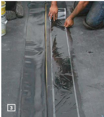
LAY IN THE TAPE. With the release paper facing up, the seam tape is placed on the lower layer of EPDM.
