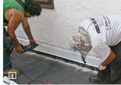
COUNTERFLASHING COMES NEXT. The crew installs a shop-formed aluminum length of nail-on counterflashing.
