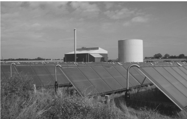
FIGURE 15.1 (See color insert.) Solar panel used for heating. The district heating station is shown in the background.
