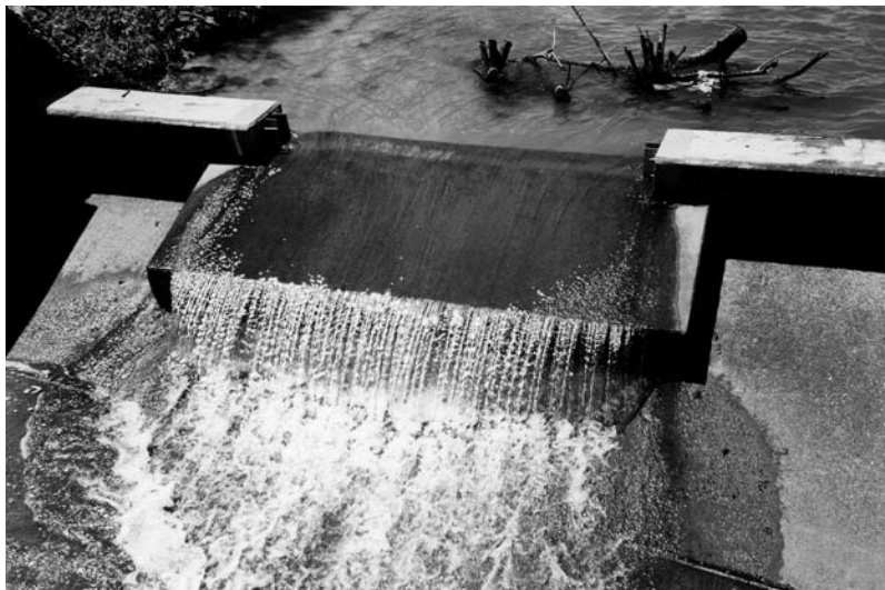
FIGURE 15.4D Close-up view of Lake Whitehurst Spillway, Norfolk, Virginia. (From Spellman, F.R., The Handbook for Wastewater Operator Certification , Technomic Publ., Lancaster, PA, 2001.)
