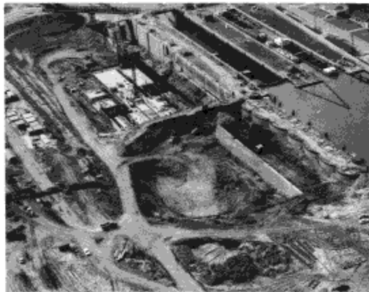
Fig. 6.27. Cellular cofferdam with berm to cut-off canal water from a large lock excavation, Canal Albert, Belgium (courtesy of Arbed)
