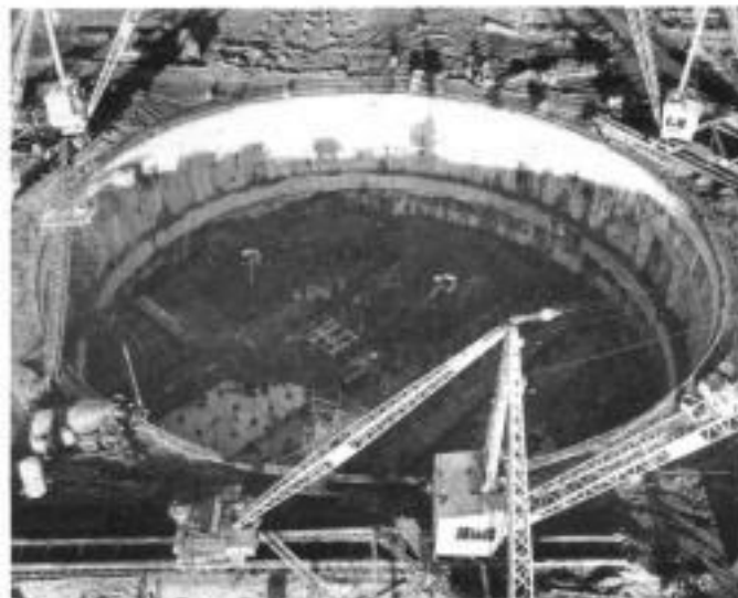
Fig. 6.4. Circular diaphragm wall with internal reinforced concrete waling, pumping station, Isle of Grain, UK (courtesy of Laing)
