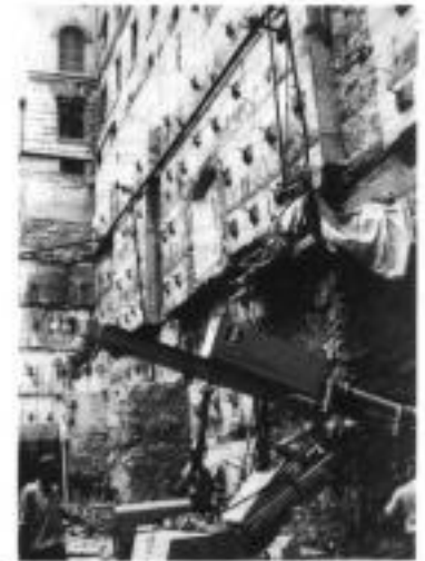
Fig. 8.4. Plate method being used for a basement extension to the Technical University, Zurich (courtesy of Bauer)
