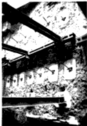
Fig. 4.3. Alternate layers of ground anchors and steel strutting used to support deep excavation between chemically-consolidated sand walls, Nuremberg (courtesy of Bauer)
