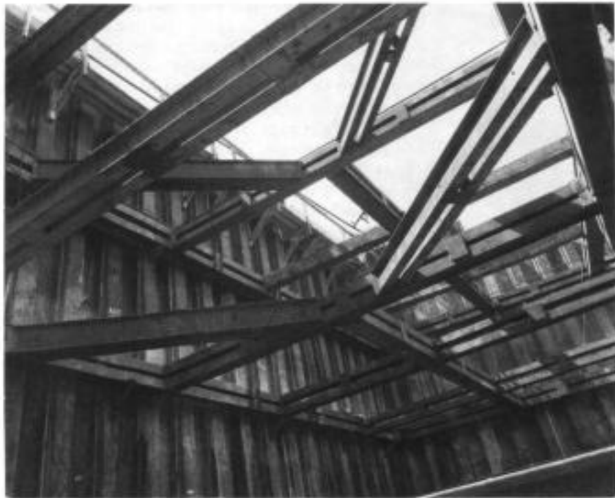
Fig. 7.23. Battened steel beams used as struts and braces on River Thames cofferdam, London
