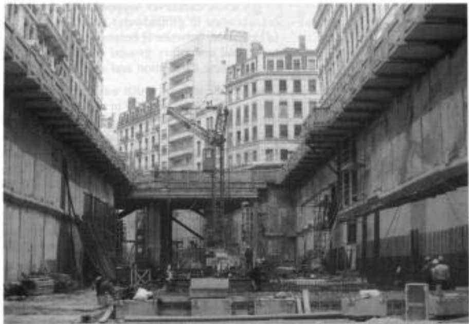
Fig. 9.34. Lyons Metro, Saxe-Gambetta station: completed station excavation showing precast diaphragm walls (courtesy of Soletanche)
