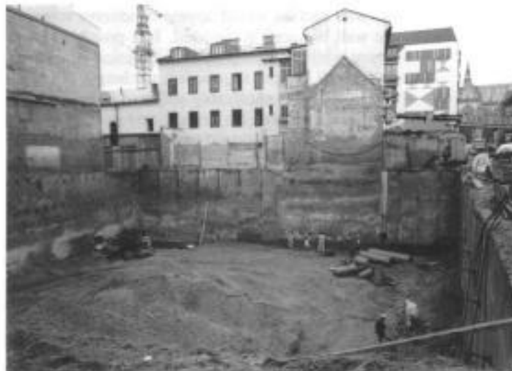
Fig. 4.34. Underpinned walls (left and centre) and walls retained by gunite overmesh between anchored steel soldiers, Linz (courtesy of Bauer)
