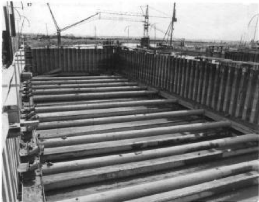
Fig. 7.22. Tubular steel struts used to brace cofferdam at Dartford Creek, UK (courtesy of AMEC)
