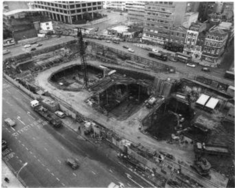
Fig. 8.10. Top-downwards basement construction with floors used as horizontal frame, Gardiners Corner, London (courtesy of Cementation)
