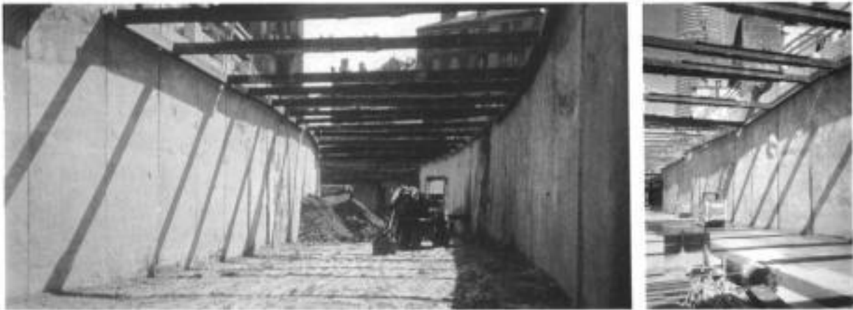
Fig. 9.37. Lyons Metro: two views of exposed precast Panosol panels in running tunnel (courtesy of Soletanche)
