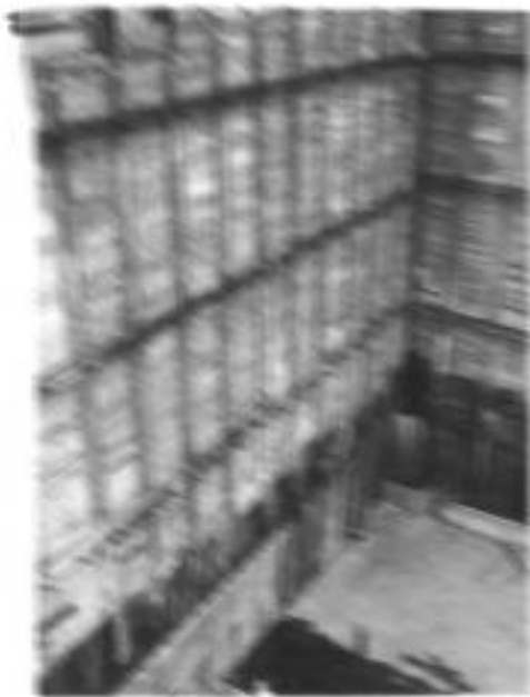
Fig. 4.4 Close placement of vertical bars and horizontal ties in concrete wall and dense reinforcement in concrete slab and downward in dense walls "bottom" slower construction of Slab.
