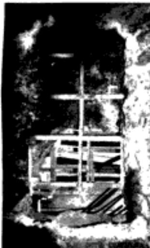
Fig. 4.23. Large mud inclusion within a diaphragm wall panel
