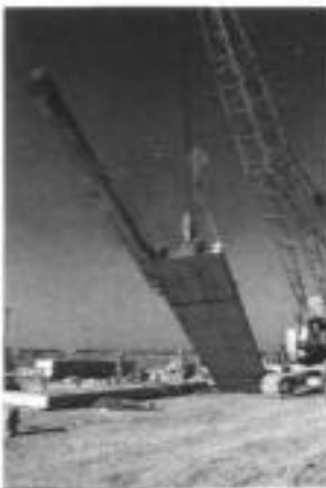
Fig. 4.25. Lifting a precast diaphragm panel at a nuclear power station at Nogent-sur-Seine, France (courtesy of Soletanche)
