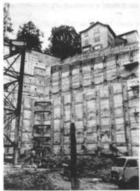
Fig. 4.7. Dual method Berlin wall for multi-storey car park, Zurich (courtesy of Bauer)
