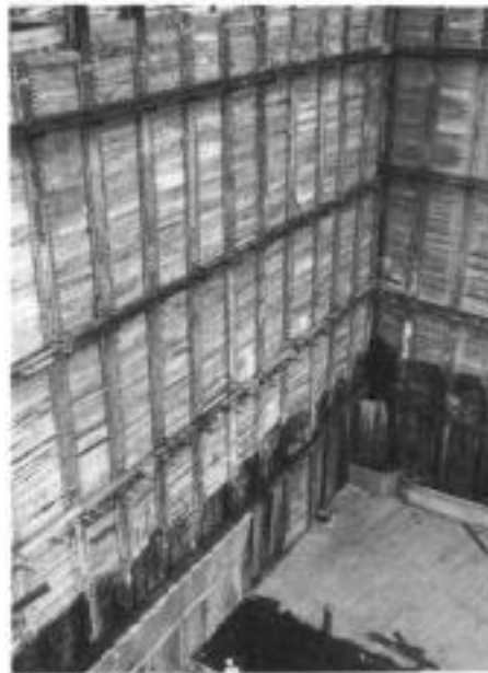
Fig. 4.6. Deep excavation through sandy silts and silty sands supported by anchored Berlin wall and dewatered by deep wells, Hannover subway (courtesy of Bauer)
