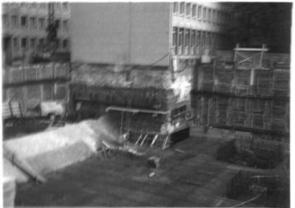
Fig. 4.3. Downward construction of Frankfurt am Main: anchored grouted wall (underpinning and anchored Berlin wall used in sandy ground without possibility of Dünung)
