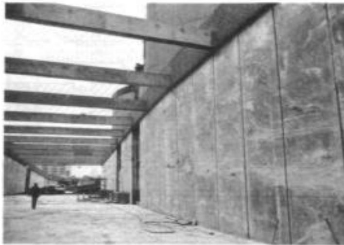
Fig. 4.24. Precast diaphragm wall construction: a high standard of wall finish is obtained using the Prefasil system, Schipol, the Netherlands (courtesy of Bachy)
