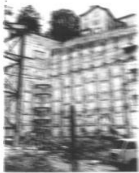
Fig. 4.5 The vertical Slab wall in full-scale of wall, Slab, columns of Slab.
