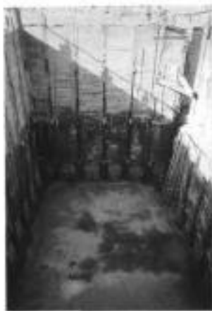
Fig. 6.21. Berlin wall method using anchors to scale pit building, depth to formation level 14 m, groundwater table at a depth of 3 m, steel plant, Jubail, Saudi Arabia (courtesy of Bauer)
