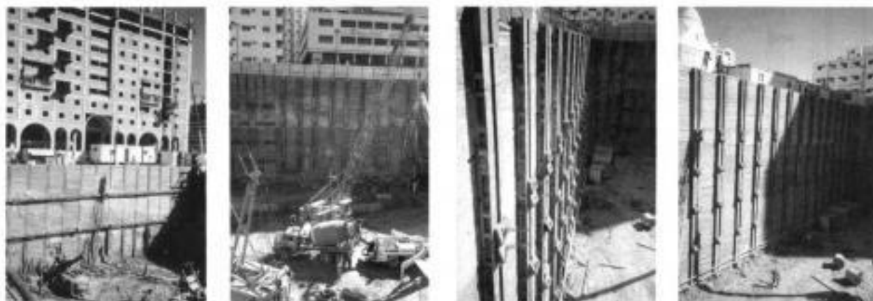
Fig. 8.15. Anchored soldier pile walls used in dry layered sand and clayey silt soil for deep basement construction. Note the unimpaired access for plant and site operations, Medinah, Saudi Arabia (courtesy of NCF)
