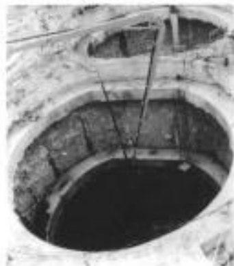
Fig. 10.5. Polygonal plan shape shaft construction using diaphragm walls, Eastern Harbour Crossing, Hong Kong (courtesy of Bachy/Soletanche)
