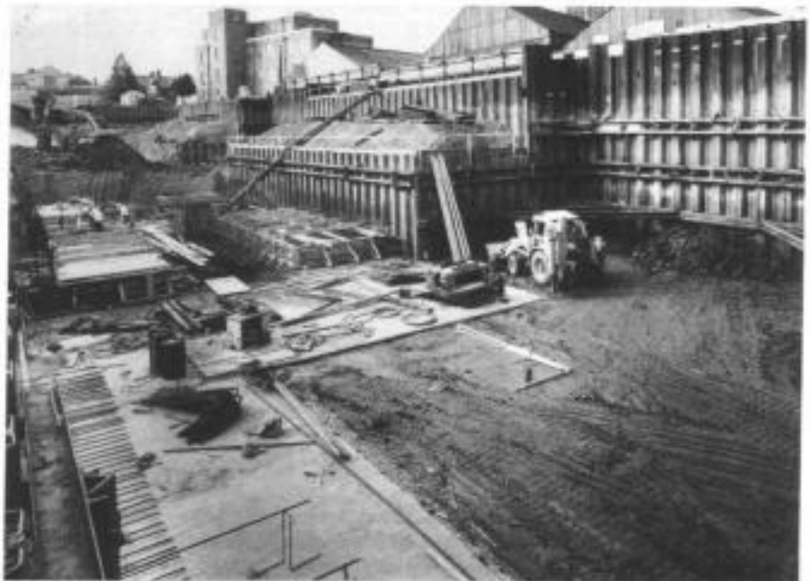
Fig. 4.9. Anchored sheet piles in London clay for a telephone switching centre, London
