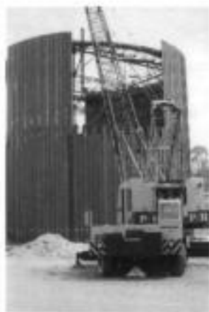
Fig. 6.38. Cellular cofferdam construction, flat sheet piles pitched and driven to a template (courtesy of Arbed)
