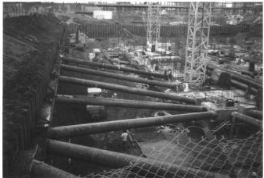
Fig. 6.1. Sheet piled excavation supported by raking shores with temporary berm support being removed by tracked excavator, London (courtesy of AMEC)
