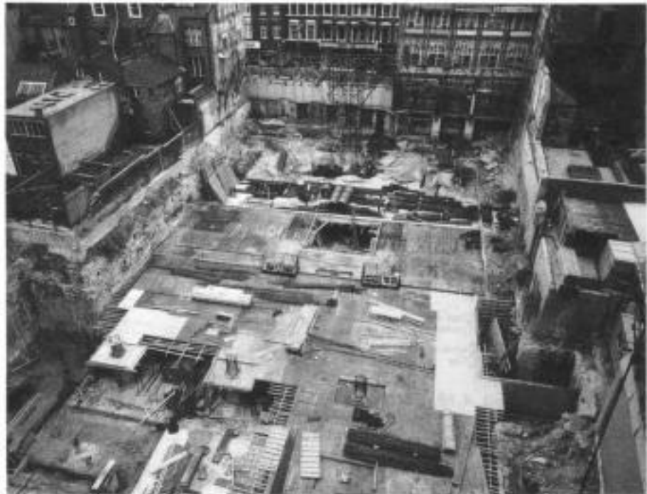
Fig. 4.18. Basement construction: diaphragm wall anchored below existing property and highway for a department store, Croydon, UK (courtesy of Lilley)
