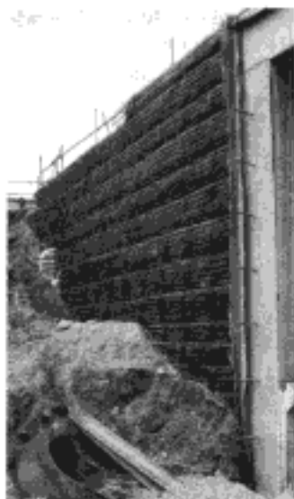
Fig. 3.1. Reinforced Earth construction to bridge abutment at trunk road improvement to A1(M) in Hatfield, Hertfordshire, UK (courtesy of Netlon)
