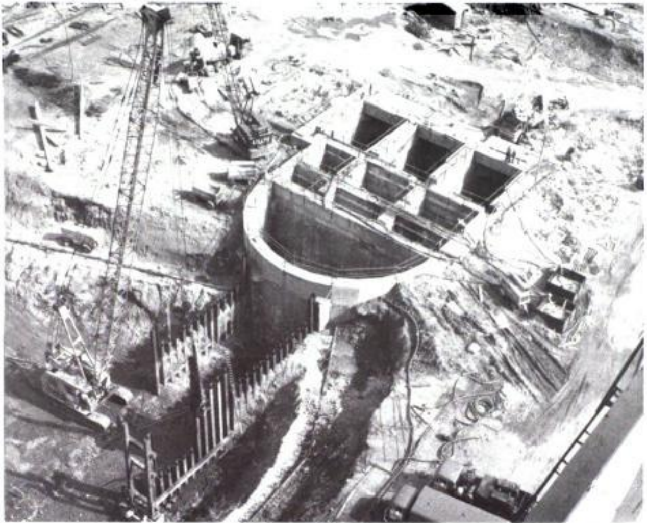
Fig. 6.25. View of construction of diaphragm wall to pump house, steelworks, Redcar (courtesy of Lilley)
