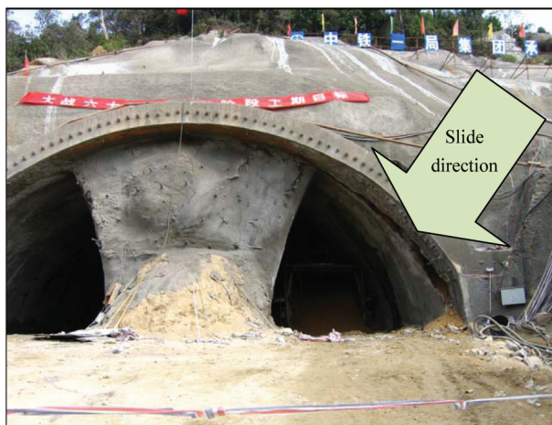
FIG. 9. First lining instability caused by landslide
