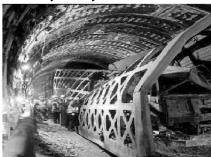
FIG.1. Fire damage to tunnel segments in Channel Tunnel fire (Kirkland, 2002).
