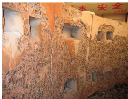
FIG. 2. Concrete spalling under high temperature. EVALUATION INDICATORS AND SAFETY STANDARD
