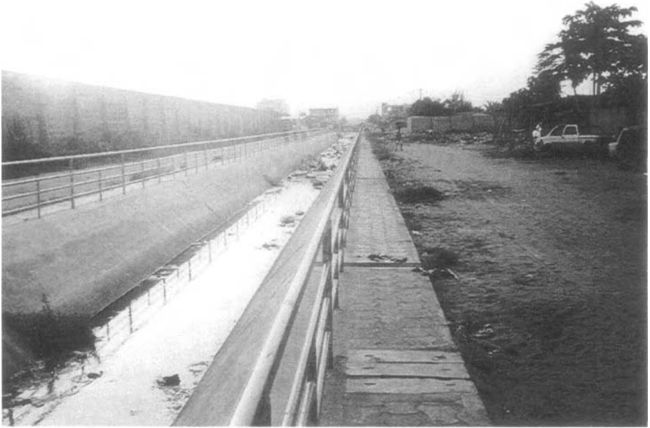
Figure 4. An open concrete drainage channel polluted with street waste.
