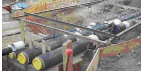
Fig. 7 Pipes for district heating cooling
