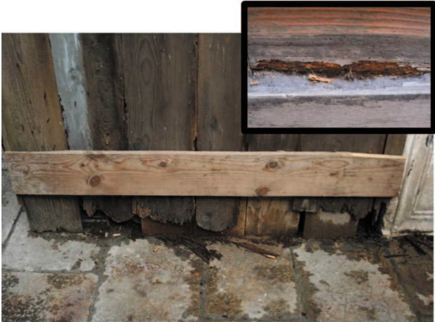
Fig. 5 Increased damages (xylophage), Venice
