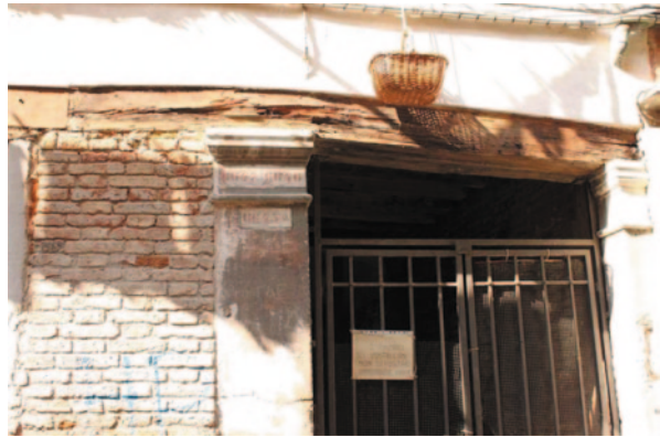
Fig. 16 Degradation by cracking, Venice
