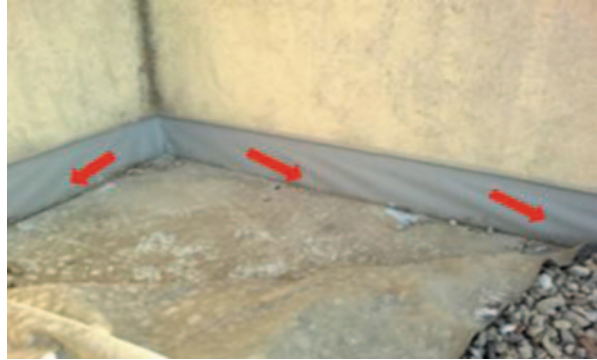
Fig. 2 South extraction area; red arrows show waves on the waterproofing, produced by loss of dimension in the lamina
