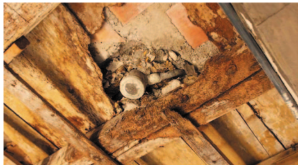
Fig. 6 Degradation by faulty plumbing in sottoportego , Venice
