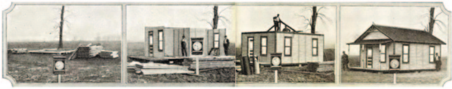
Fig. 1 Sears Simplex, process of erecting in 8 h. (Source: Sears Modern Home Catalog, 1921)
