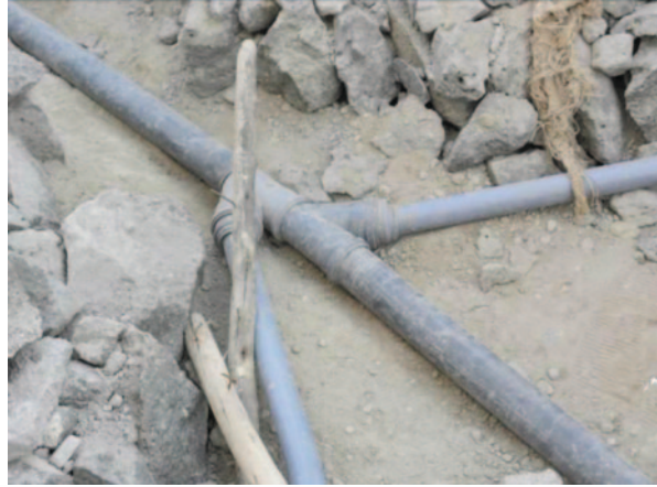
Fig. 6. Detail of water distribution pipeline. Photo by author
