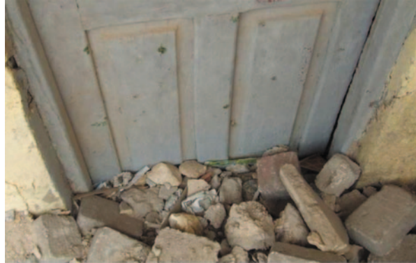
Fig. 4 Obstruction of lower part, Dakhla
