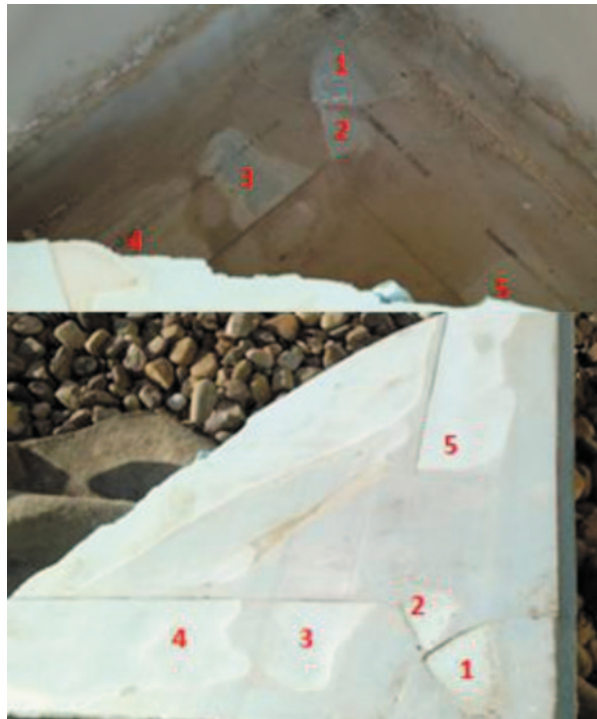
Fig. 3 South extraction area, in the superior part the PVC-P lamina, in the inferior part the XPS board, red numbers identify interactions
