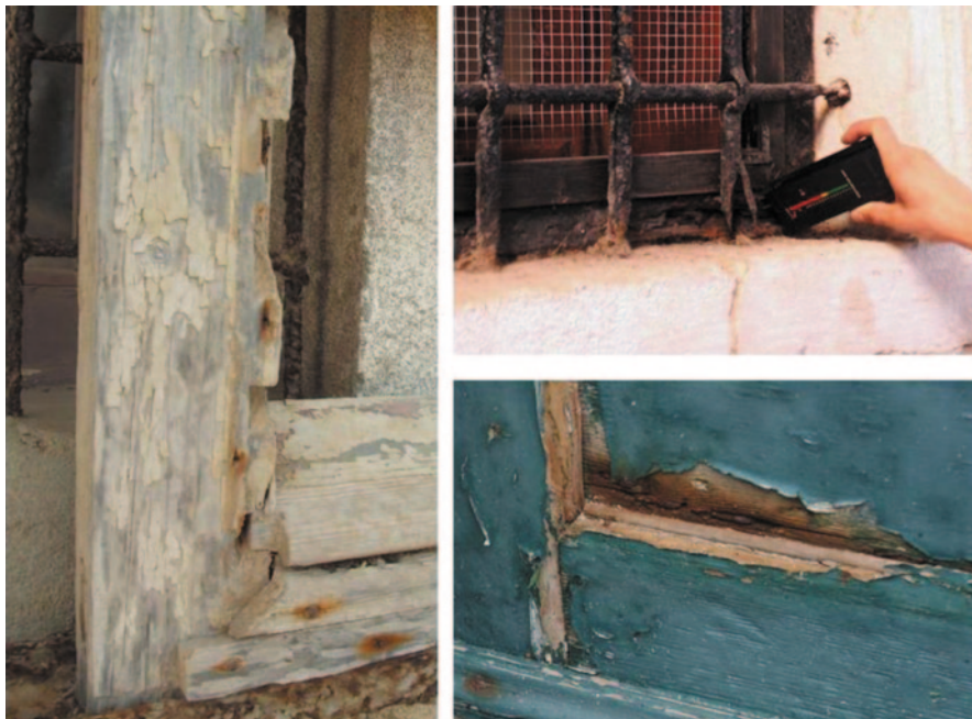
Fig. 14 Degradation by ferrous elements, Venice
