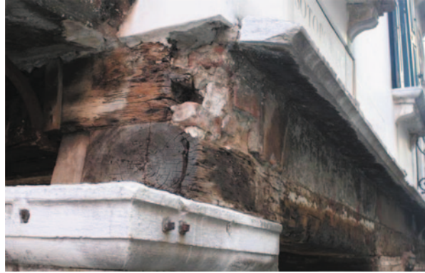
Fig. 18 Degradation by lost of material, Venice
