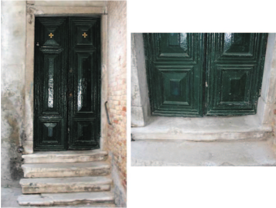
Fig. 17 Degradation by differential thrust, Venice
