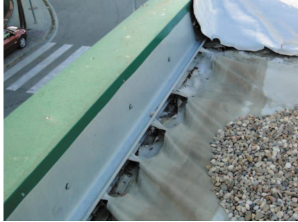
Fig. 4 Loss of plasticizers in a PVC-P waterproof membrane, showing consequently a considerable shrinkage of the sheet. (Source: GEORA Aplicaciones Técnicas)
