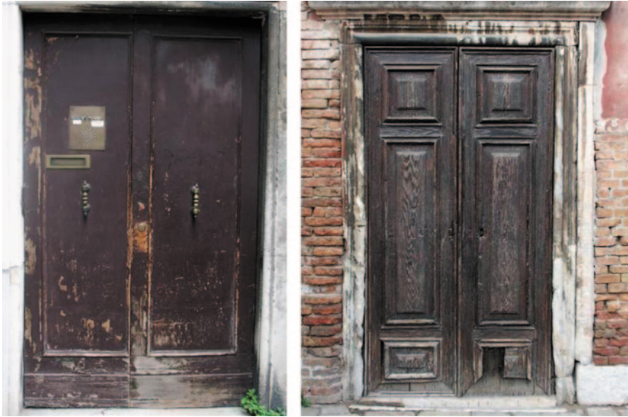
Fig. 10 Degradation by absence of hinge maintenance, Venice
