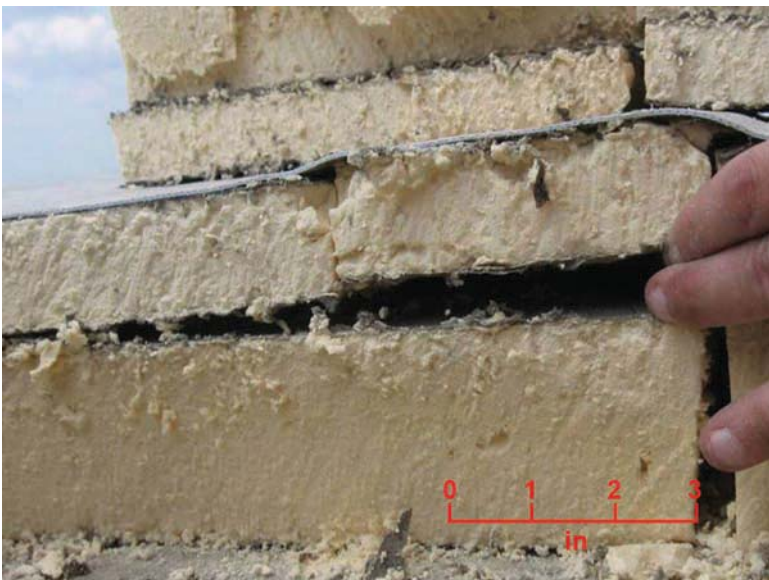
FIG. 8—Curled-up edges of the insulation boards were no longer adhered to the insulation below.
