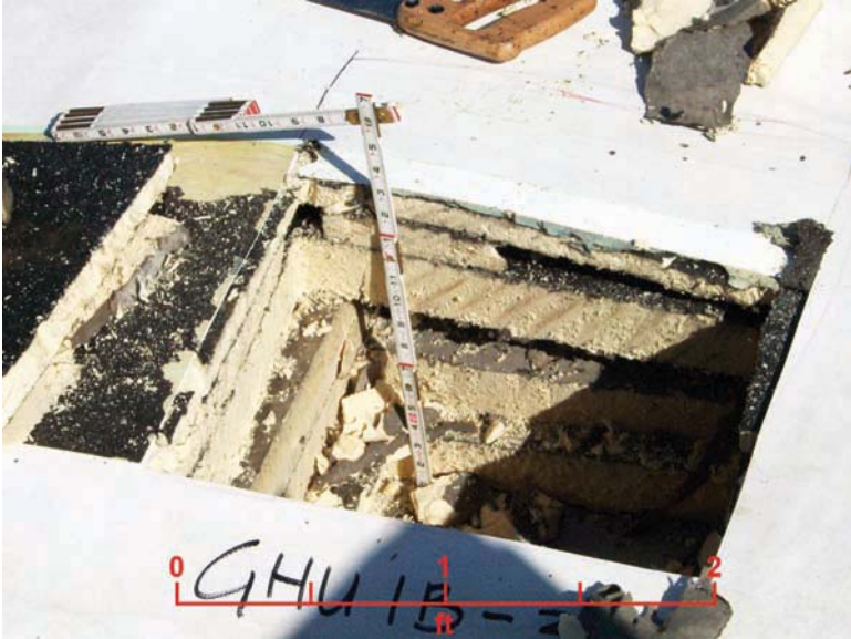
FIG. 7—Displaced insulation boards within the roofing assembly below the TPO membrane.
