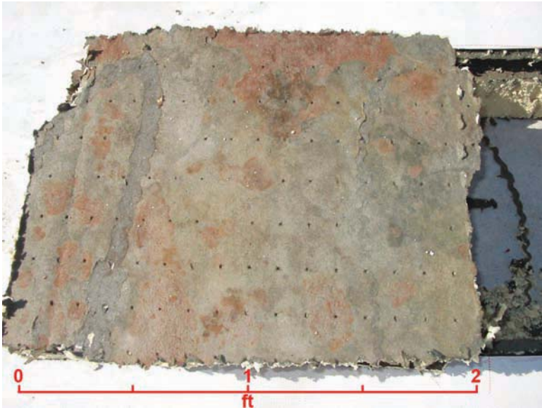
FIG. 5—Significant staining and signs of biological growth on the bottom layer of an insulation board facer.
