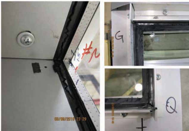
FIG. 15—Typical structural sealant damage.
