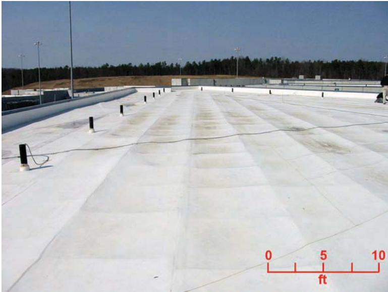
FIG. 2—Notable insulation board deformation reflected through the TPO membrane.
