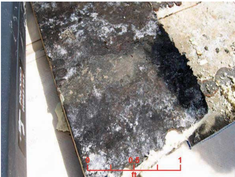
FIG. 6—Apparent microbial growth on an insulation board facer.
