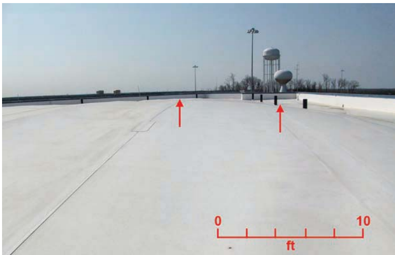
FIG. 1—TPO roofing membrane inflation and billowing.
