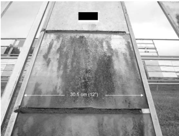
FIG. 30—Acrylic terpolymer sealant #11, before cleaning.
