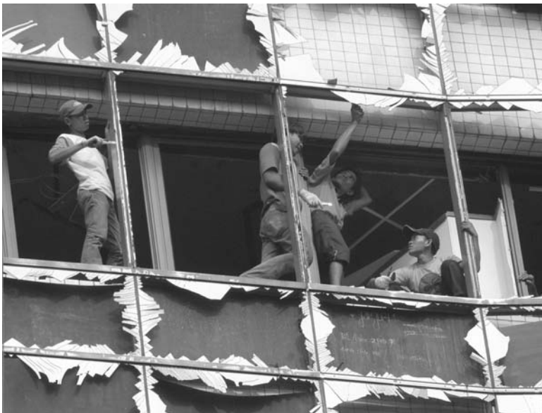
FIG. 1—Glazed curtainwall damaged by bomb blast (note the remaining shards of glass) (Source: Associated Press).
