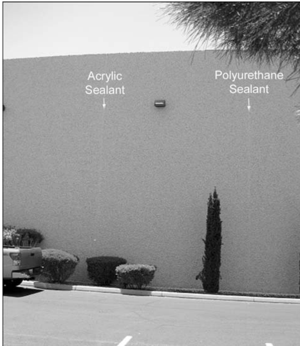
FIG. 3—View of the east elevation of the El Paso warehouse with an acrylic sealant joint on the left and a polyurethane sealant joint on the right.
