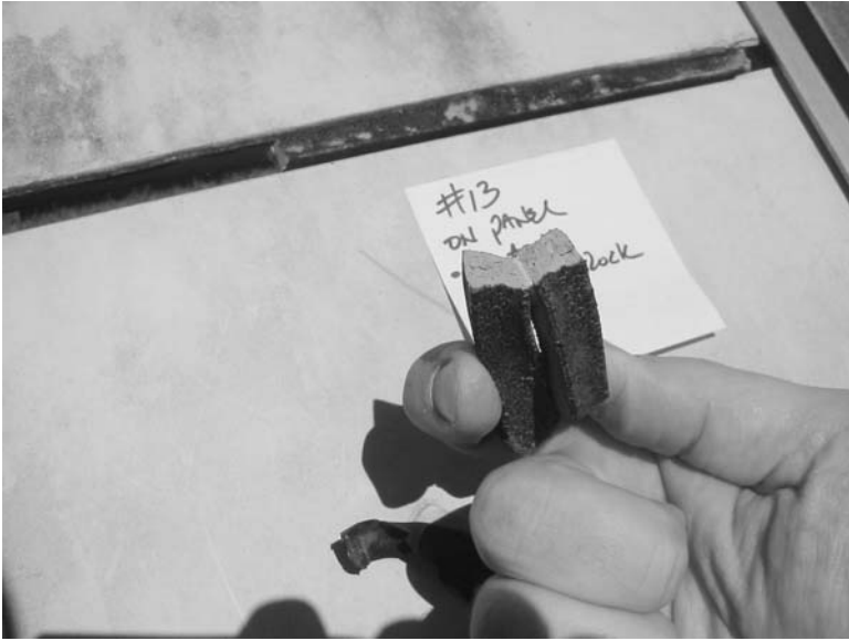
FIG. 8—180° manual bend of sealant (rated Poor).
