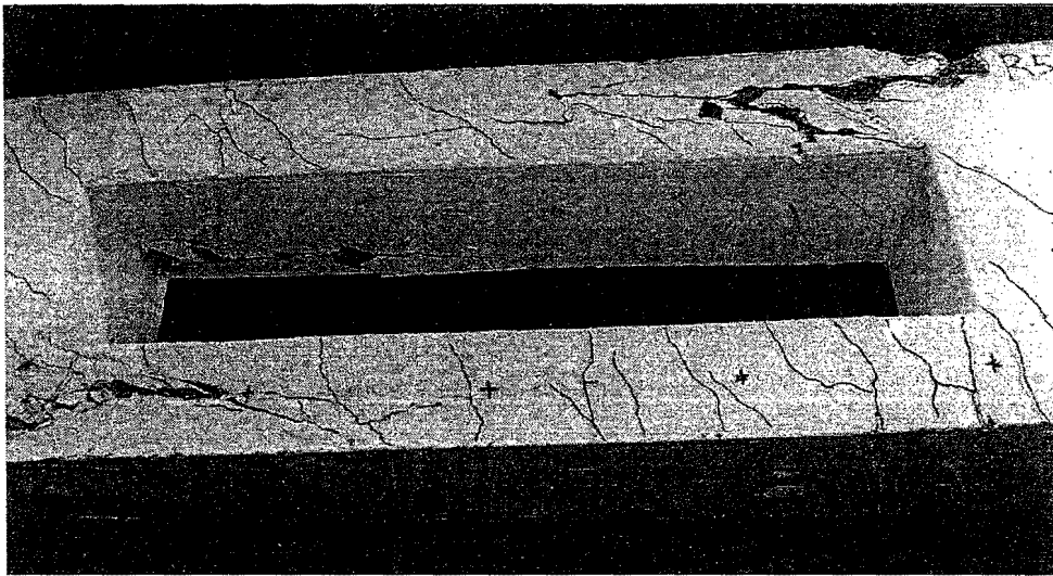
Figure 4.1 Typical mode of failure of a beam with large rectangular opening under predominant torsion.
