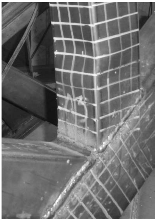
Figure 6. Failure in a 55° K-joint without vent hole.
