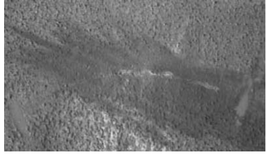
Figure 8. Crack in the grout repair node: no indication of growth since repair.
