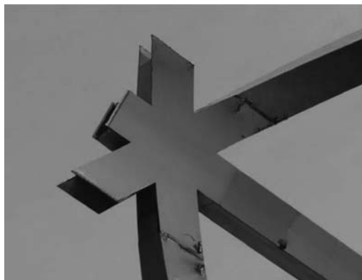
Figure 10. “Star” under construction on site, with two diagonals and one chord waiting to be connected.
