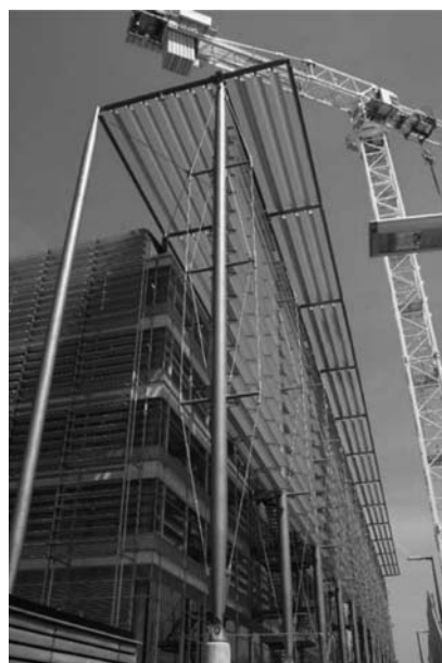
Figure 2. Prestressed stayed tubular column in the Chiswick Park development in West London, UK.
