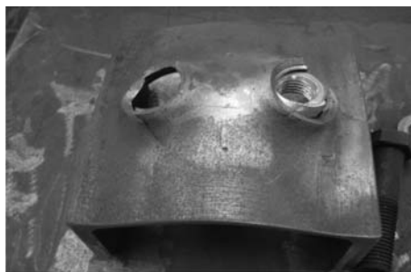
Figure 7. RCT1, Web cracking.
