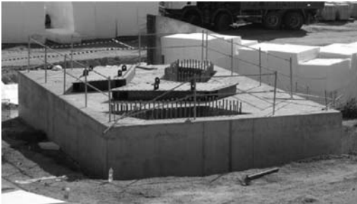
Figure 12. General view of a pile cap concreted, with the reception chambers with connecting bars, and the pinned-fixed connection elements waiting to be inserted, on top.
