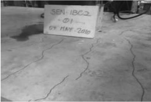
Figure 6. Fine cracks appeared close to column.
