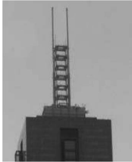
Figure 3. Cracking in tubular discovered by lighting technician.
