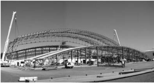
Figure 19. Award winning post-tensioned aviation hangar with a 78 m clear span erected with minimal assembly time.
