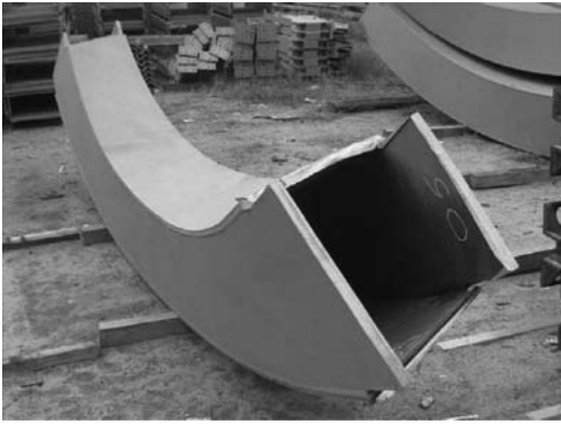
Figure 17. A diagonal finished with its ends prepared to be welded against two stars.
