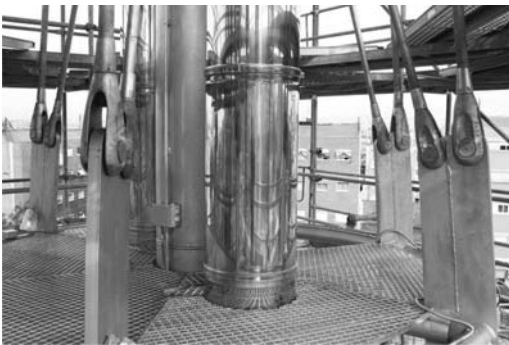
Figure 16. Transition plate where braces are fixed.
