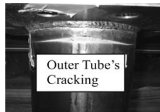
Figure 7. Cracking of tensile region.
