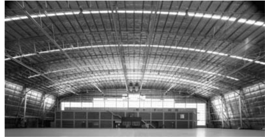
Figure 5. Aircraft hangar, with an 84 m clear span, constructed through the implementation of the post-tensioning technique.
