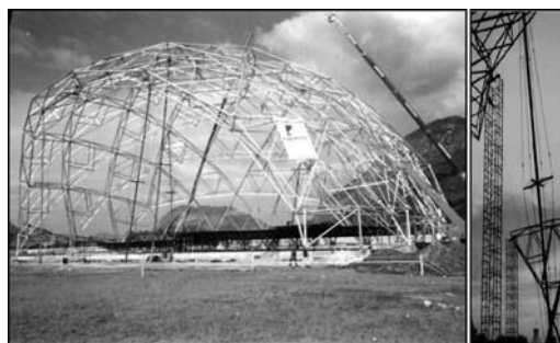
Figure 1. Real structure being erected with prestressed carbon steel stayed column (Andrade et al. 2003a & 2003b).
