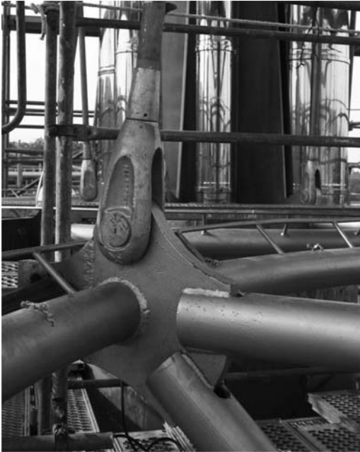
Figure 15. Transition plate where braces are fixed.
