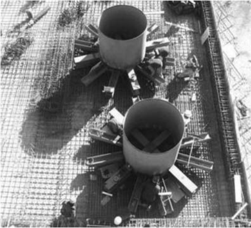
Figure 11. Metallic profiles designed to transmit stresses from the shaft to the concrete slab.
