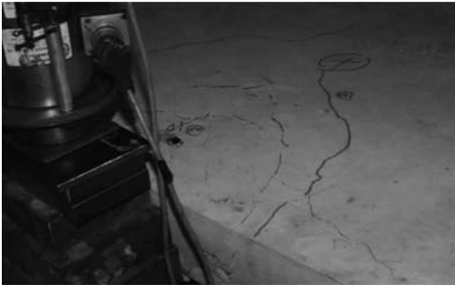
Figure 7. Cracking at the end of concrete slab.
