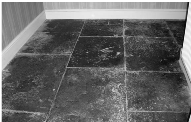
Photo 4.1 Special care is needed when lifting stone flags to rebed on an insulated floor
