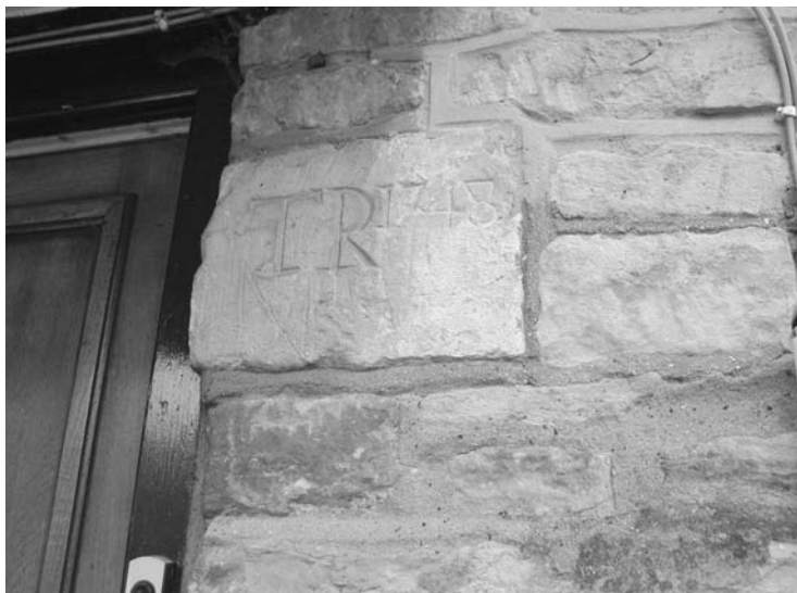
Photo 4.3 Poor cement mortar repointing, preceded by even earlier poor repointing adjacent
