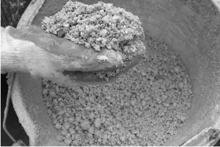
Photo 7.32c Limecrete floor technology – lightweight pumice and lime ready to be laid on to the sub-base of foamed glass
