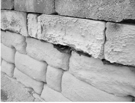
Photo 7.9a Salt crystallisation – wind-driven salt erosion is worse in softer stone beds
