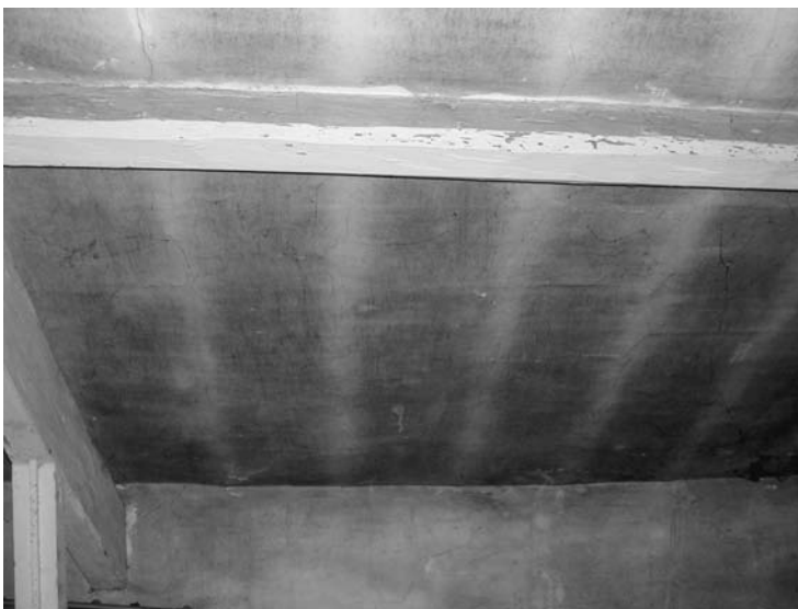
Photo 4.6 A bad case of black mould due to condensation on the cold areas between the wooden joists
