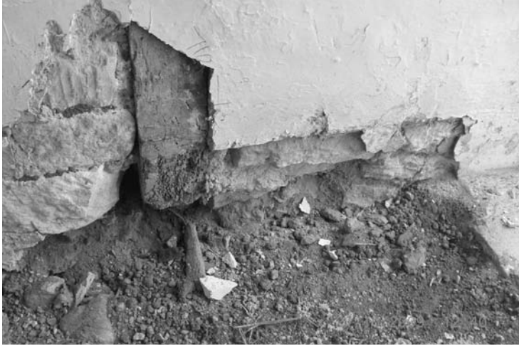
Photo 3.1 Footings absent in a 17th-century house due to 19th-century excavations to lower the floor
