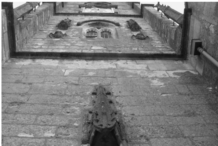
Photo 7.7b Calcium sulphate decay in a much larger sheltered area
