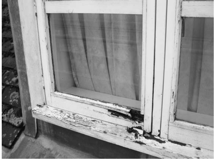
Photo 7.1 Wooden window left to rot in the expectation of replacement with UPVC
