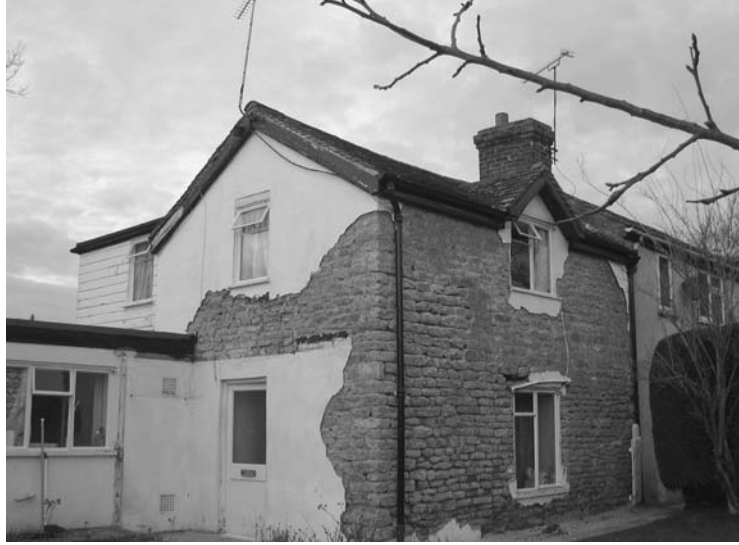
Photo 7.28 Cement render can rarely be totally removed
