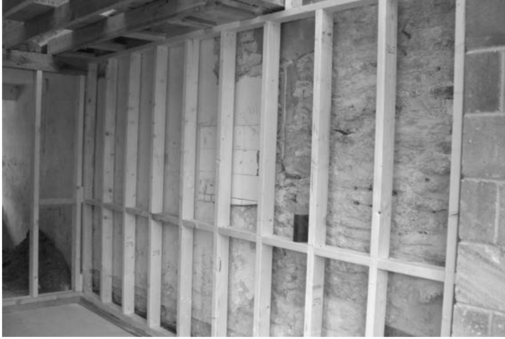
Photo 4.28 Drylining being installed over a traditional stone wall – the timber should have been isolated to avoid the danger of dry rot
