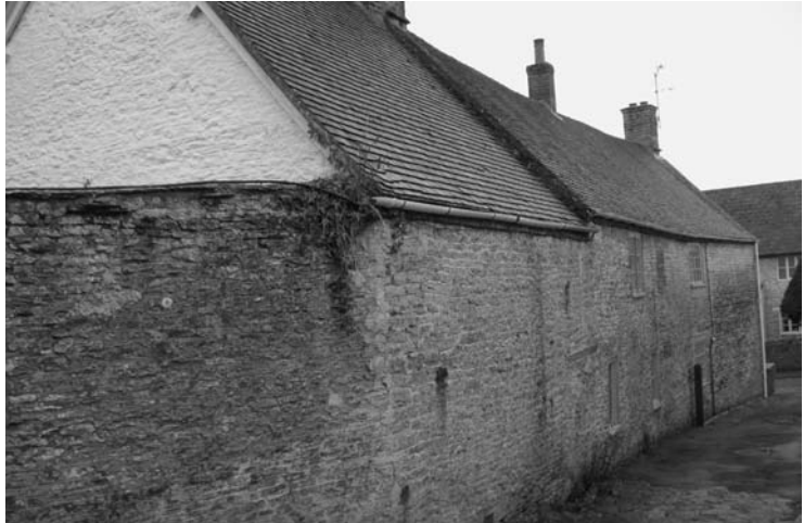
Photo 7.4f Vegetation at gutter level is a sure sign of major repair problems in the future
