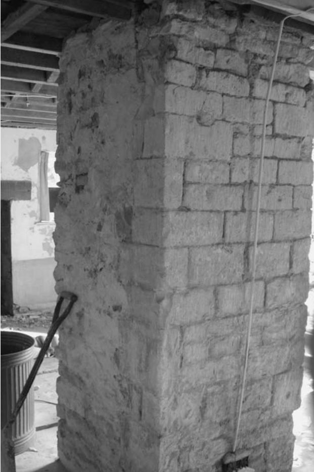
Photo 3.9 Regular stonework on this newly revealed chimney, now buried within a house
