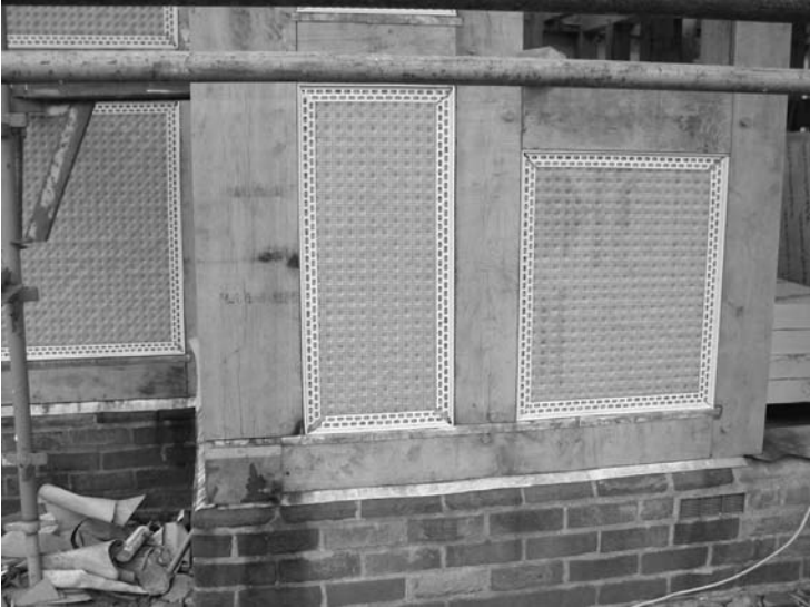
Photo 6.14 Detail of treatment of panels in the new traditional timber framed house, showing sheathing to take render, also lead as a damp course which may well be leached due to tannic acid from the oak
