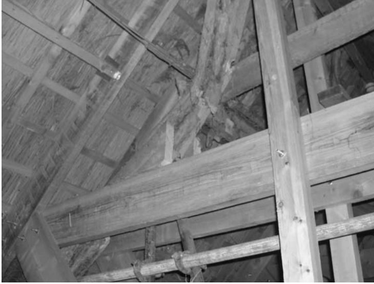
Photo 6.35 A traditional roof has lost its meaning in a welter of new support timbers and is in danger of needing to satisfy Building Regulations for a new roof
