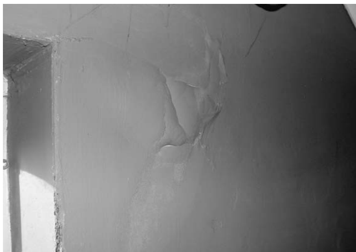
Photo 4.9 Internal gypsum plaster exploding due to water ingress from an exposed external gable elevation facing across a valley
