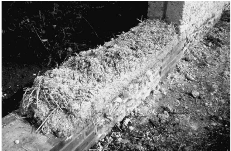
Photo 7.31c A new cob wall being constructed in lifts, re-using old cob chopped up with straw and water
