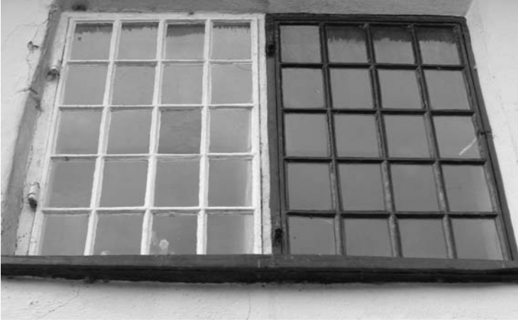
Photo 5.10 Historic metal casements with pintle hinges deserve to be retained and secondary glazed
