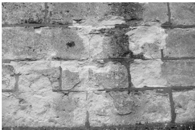
Photo 7.7c Calcium sulphate decay – the cement pointing is accelerating decay by forcing more wetting and drying cycles to take place in the stone
