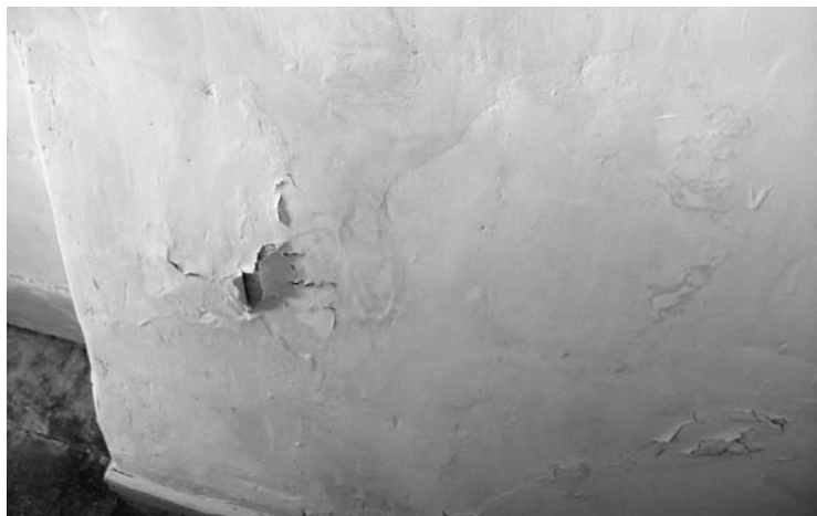
Photo 7.11 Rising damp reaching an evaporation zone affects internal finishes; an externally sited French drain can do much to alleviate this problem
