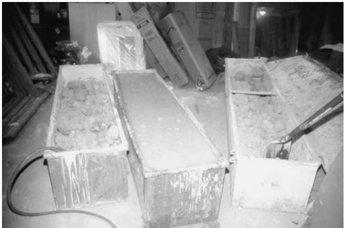
Photo 2.20 The slaked lime is ready for combining with sand to make a mortar or rendered mix
