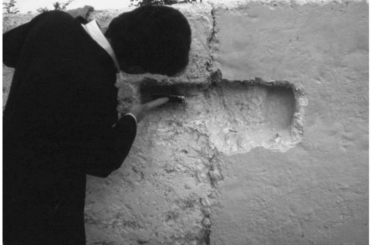
Photo 7.31b A crack in a cob wall can be repaired by stitching across the deliberately created ledge with cob bricks or flinging handfuls of cob to fill up the gap
