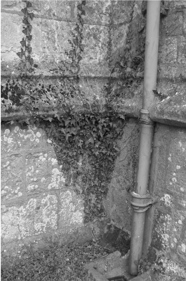
Photo 7.3 The clearing of gullies and checking of downpipes for blockages is fundamental for all types of construction; here ivy is also a problem and needs to be kept under control
