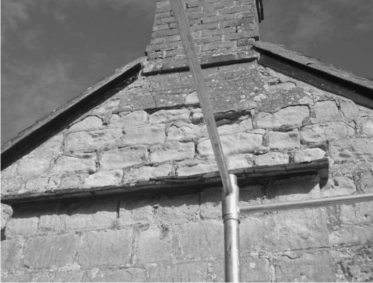
Photo 7.12 Calcium sulphate decay always occurs at the base of chimneys where hot sulphur-laden gases impregnate the stonework, altering the chemical state of the stone; rendering in cement exacerbates the problem, holding in water to further mobilise salts
