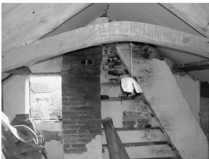
Photo 7.4d Years of neglect of a chimney flashing for want of minor works, evident in the poor condition of this chimney breast
