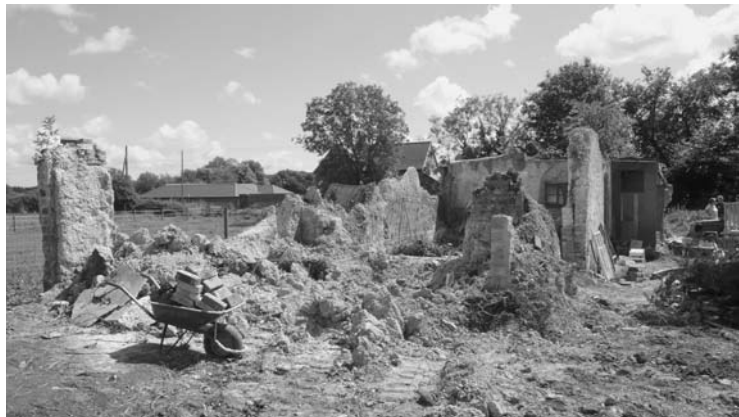
Photo 6.10 Cob barn prior to reconstruction using the existing material (photo © Rob Buckley)
