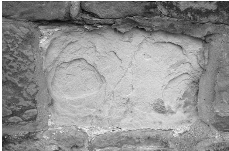
Photo 7.10 Contour scaling on sandstone
