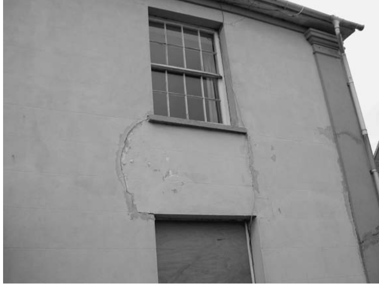
Photo 2.52 Cracks in cement render caused by expansion of brick substrate
