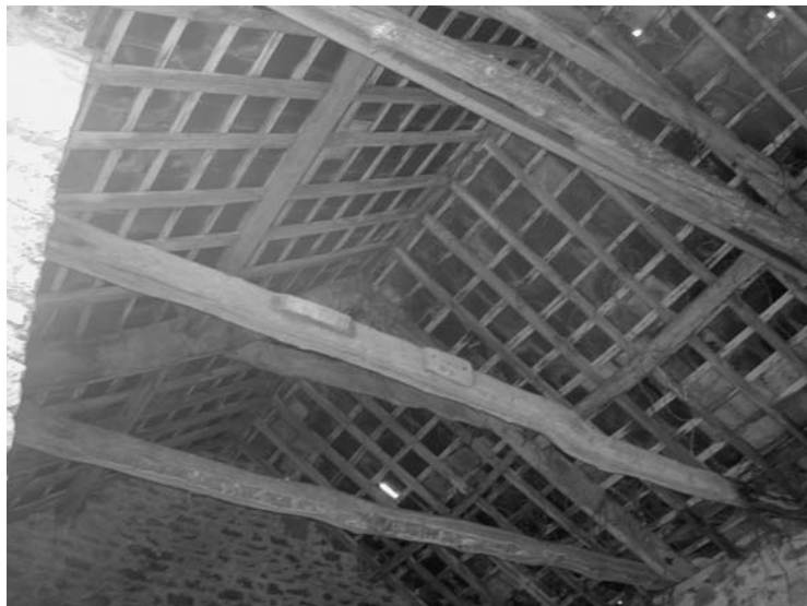
Photo 5.20 Proposed barn conversion – untouched roof ideal for incorporating high levels of insulation above the rafters without disfiguring the roof construction
