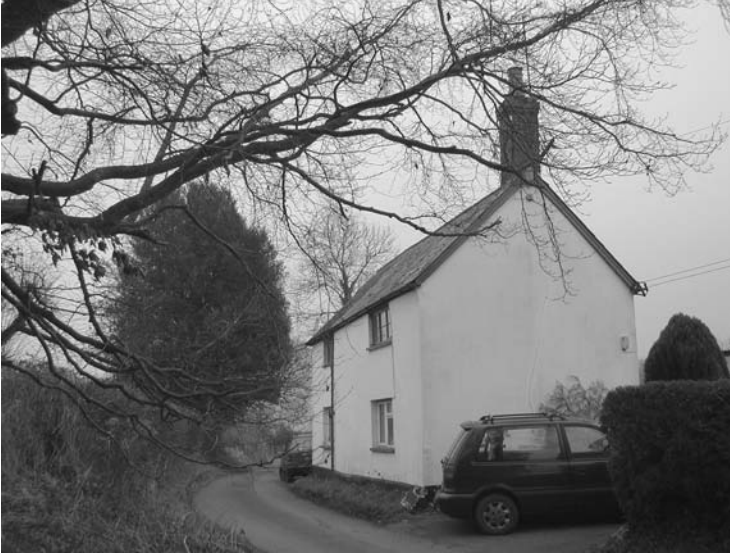
Photo 2.9 Dorset cob house rejected because the gable needed rebuilding
