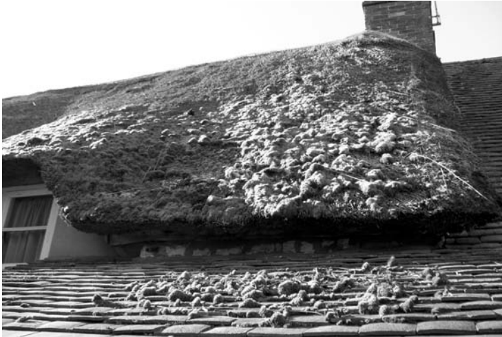
Photo 3.30 Moss on a thatched roof means it is no longer functional
