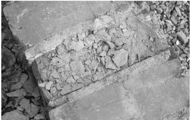
Photo 7.25 Frost action on garden path exacerbated by ground-driven salts
