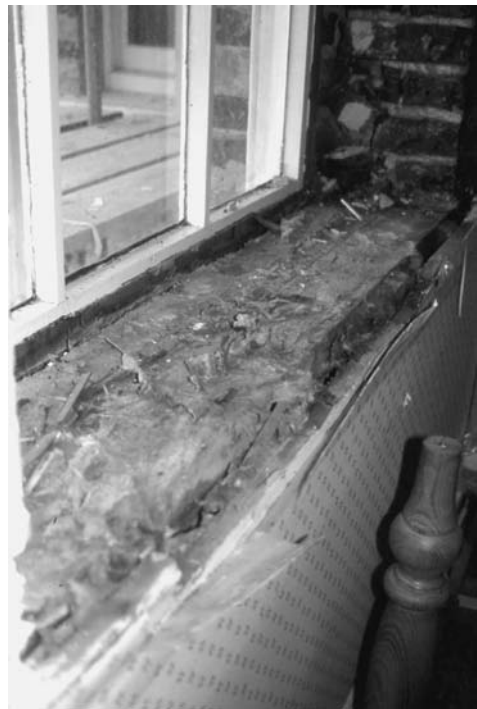
Photo 7.19 Desiccated dry rot on a cill in a Georgian building
