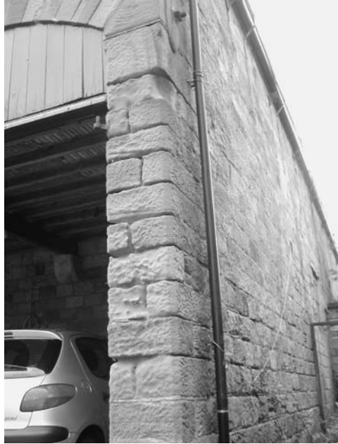
Photo 7.9d This stone pillar is graphically illustrating salt erosion in an exposed location
