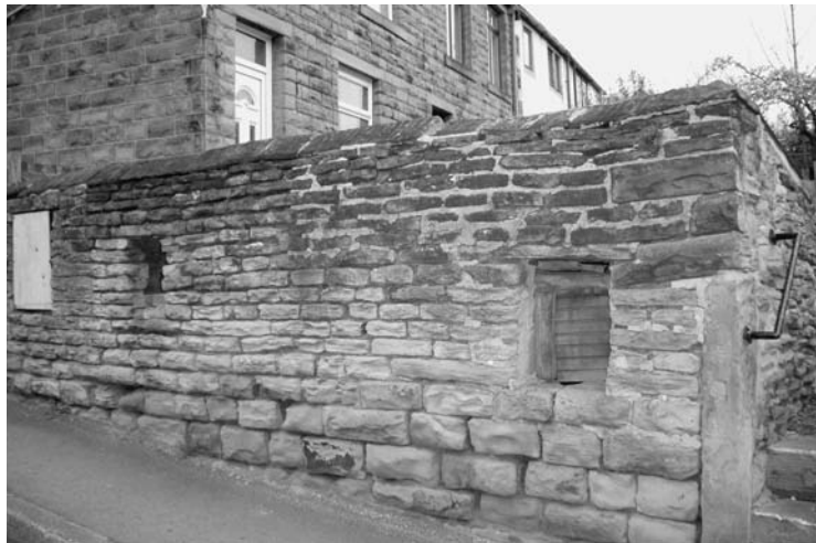
Photo 7.4a Former pigsty in West Yorkshire has suffered many years of neglect and variable minor works, just enough to ensure its survival
