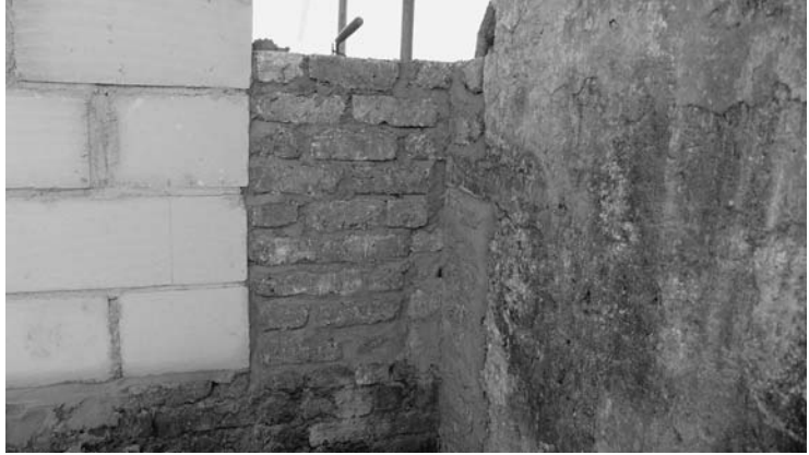
Photo 7.31a Cob repair using unbaked bricks to join an existing cob wall to a blockwork wall (photo © Rob Buckley)
