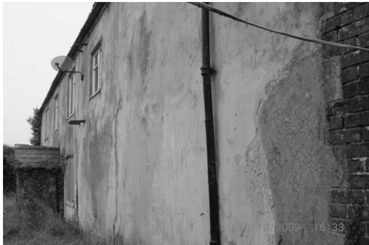
Photo 7.14 Cracks in cement render due to expansion of the stone underneath – it needs replacing with lime render, a more permanent but still sacrificial overcoat
