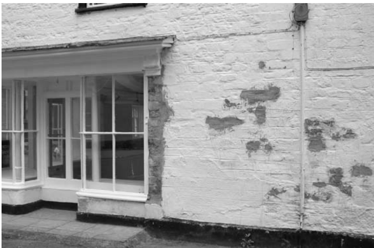
Photo 7.27 Patching old stone walls with cement is a recipe for further decay
