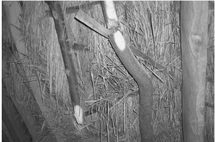
Photo 2.29 Pole rafter roofs can sometimes fail but can be replaced if there is a thriving coppicing initiative
