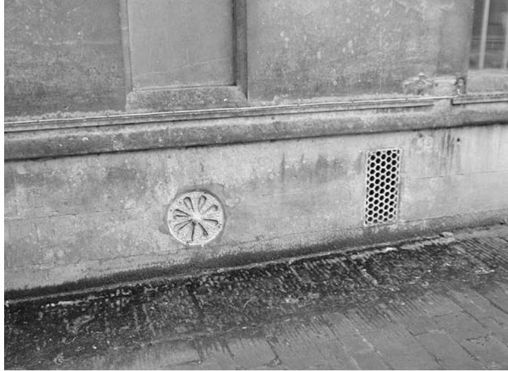
Photo 4.22 Manual ventilation controls at Victorian Tynesfield House, near Bristol
