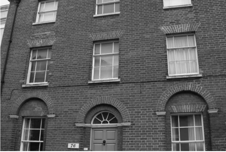
Photo 7.29 Cement pointing on gauged brickwork has fortunately not extended to the brick arches, or as yet caused much decay overall
