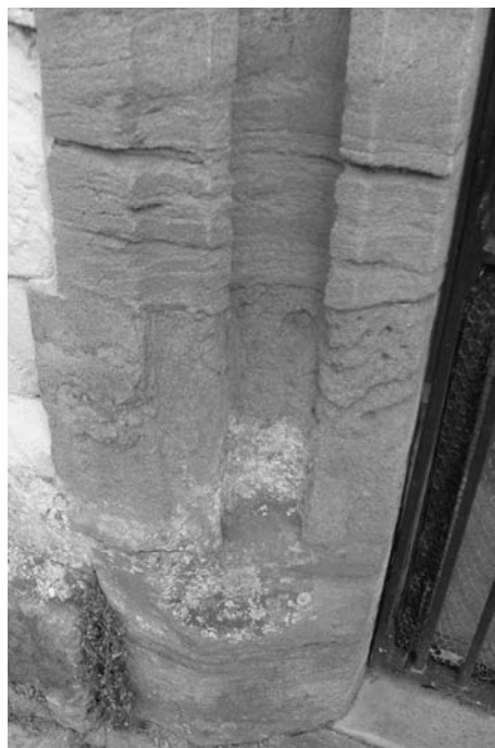
Photo 2.4 (right) Yellow Hamstone panel at the base of a church doorway suffering from salt erosion
