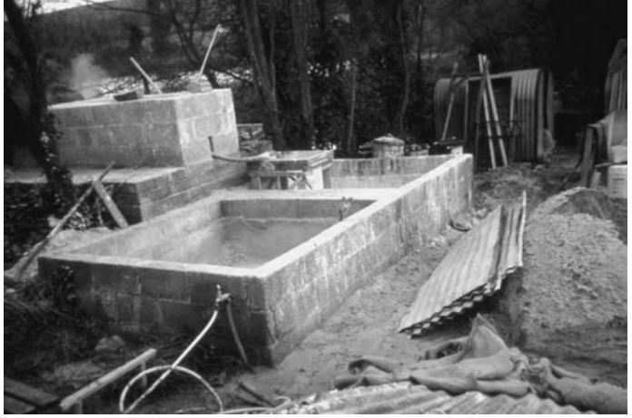
Photo 2.18 Burnt limestone is slaked to form lime putty in a lime pit
