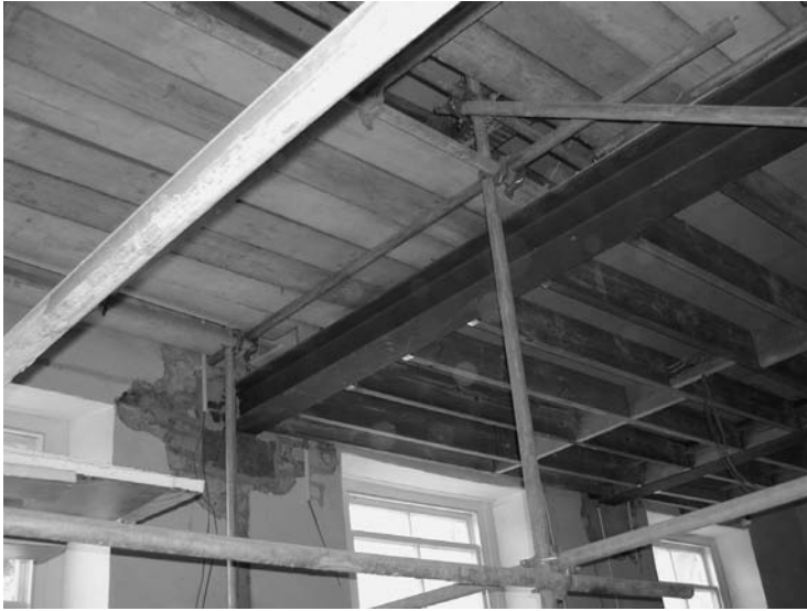
Photo 6.26 Steelwork inserted into a traditional building possibly has only a limited lifespan compared to the already great longevity of the existing building.
