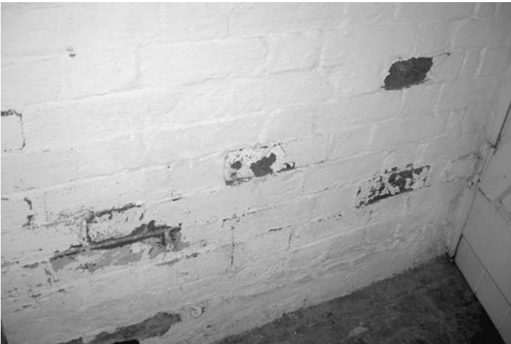
Photo 7.13 The salts in the base of this internal brick wall need to be poulticed out
