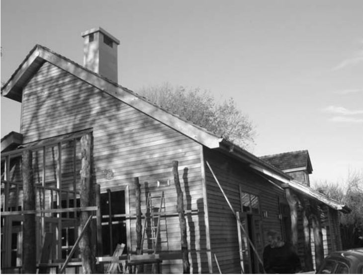
Photo 6.29 Another view of the boarded timber frame building near Weymouth during construction
