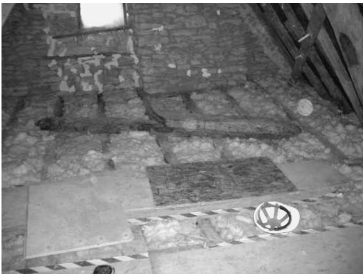
Photo 4.10 Loose sheep's wool insulation being laid in a 17th-century roof (photo © Rob Buckley)
