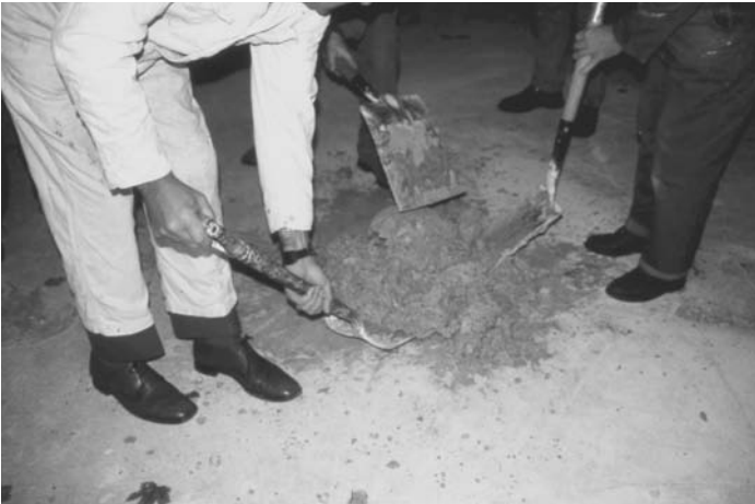
Photo 2.23 Mixing can be done by cutting and slicing the lime putty into the sand
