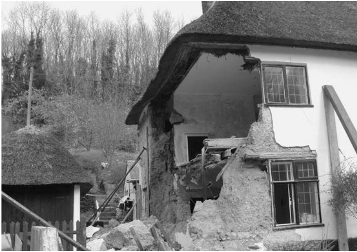
Photo 6.6 Partial collapse of a building at Milton Abbas, Dorset
