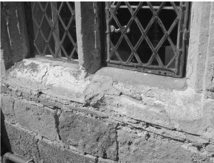
Photo 7.16 Unfortunate cement repair of previous salt-eroded stonework on this precious mullion window is actually causing further erosion
