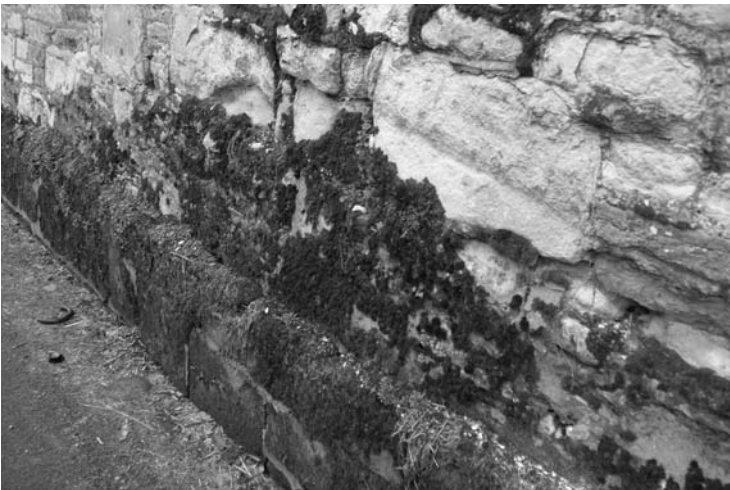
Photo 7.6 Moss is a sign of continuously wet masonry, the drier zone above it is showing calcium sulphate erosion
