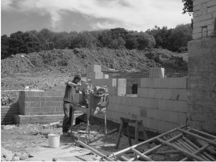
Photo 4.21 Ziegel blocks being used to line a stone wall in a new extension to a traditional building
