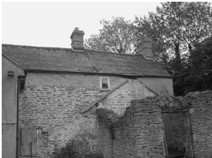
Photo 3.20 Fishscale roof tiles on a clay-mortared Dorset farmhouse; they were also used as wall cladding
