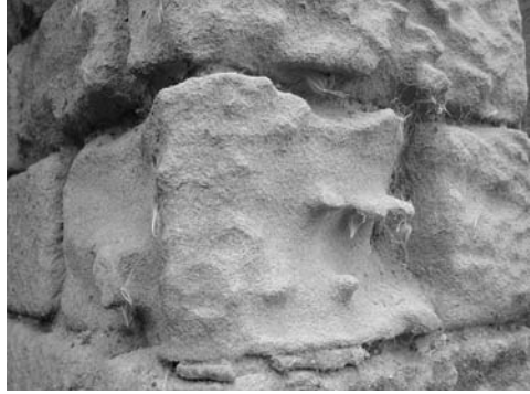
Photo 7.9c Salt crystallisation – corners of stonework are particularly prone to wind-driven salt erosion as they are evaporation zones for water
