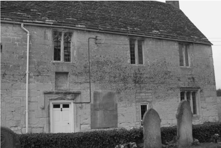
Photo 7.5 Lichen is concentrated in the middle wet zone whilst decay is concentrated in the lower zone due to rising and mobilised salts
