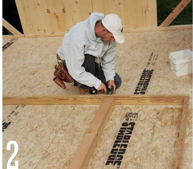
2 Build the timber-panel wall frame out of 2×4s. Then, fasten a 4×4 post in between the top and bottom wall plates with 3-in. screws.
