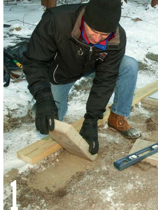
Set the solid-concrete blocks into place, then check them for level. Use a long, straight 2×6 to align each row of five concrete blocks.
