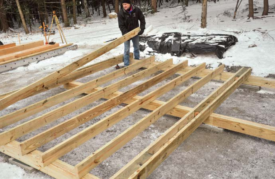
This skid foundation is built with three timbers, or skids, set on grade. The 2×6 floor joists are then laid across the skids spaced 16 in. on center.
