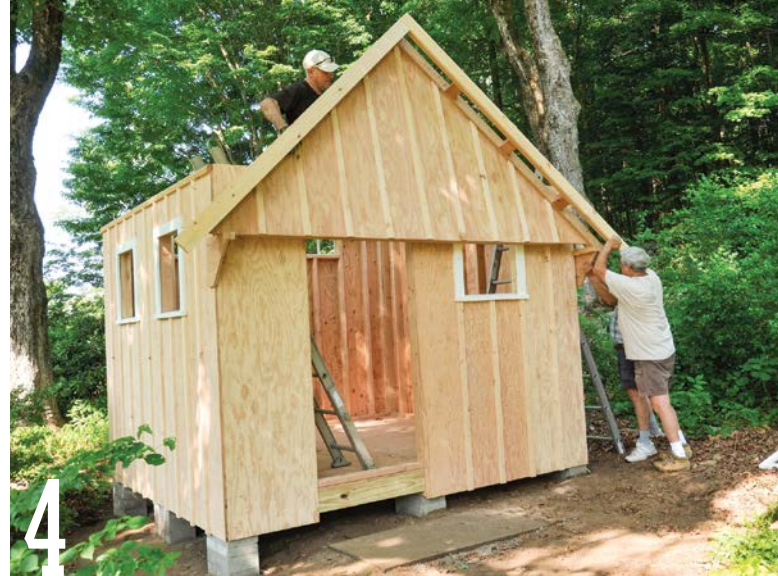
When the truss gets to within 12 in. or 16 in. of the top of the wall, lift it off the resting cleats and set it down on top of the 2×4 wall plate.
