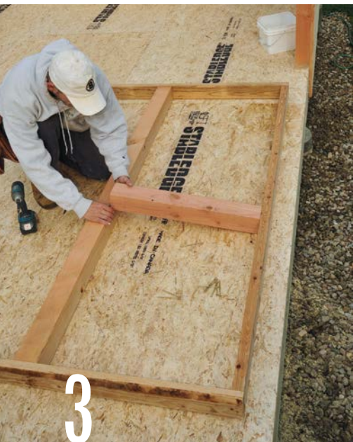
3 Cut a 4×4 purlin to fit between the 2×4 end stud and 4×4 post. The purlin strengthens the wall and provides nailing support for the pine sheathing.
