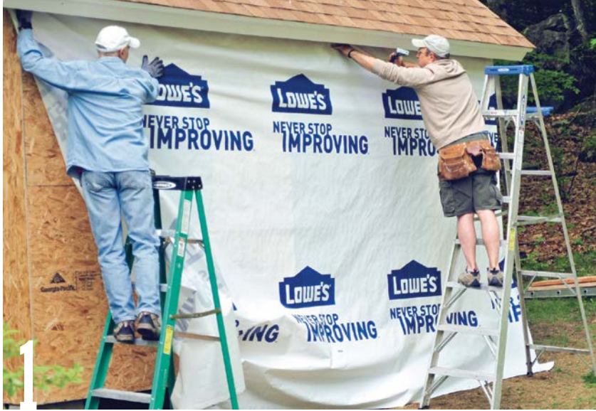
1 Cover the shed walls with housewrap. Staple the wrap to the sheathing, then slice the wrap from the vent, window, and door openings.
