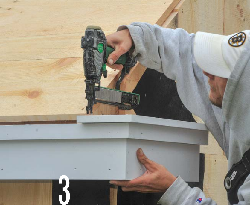
Nail a PVC cap on top of each cornice return. Cut the cap to extend \frac{3}{4} in. beyond the narrow fascia trim nailed to the fascia board.
