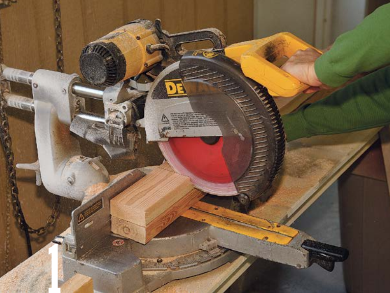
1 Use the miter saw to simultaneously cut two 2×4 wall plates. Gang-cutting multiple parts saves time and reduces measuring mistakes.
