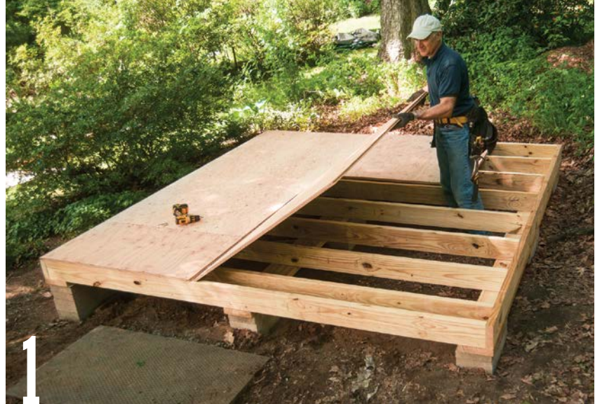
Lay 3/4-in. tongue-and-groove plywood over the floor frame. Tap the sheets together and be sure that all end joints are centered on a joist.
