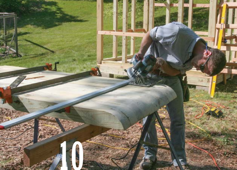
Saw the bird's-mouth cut in two passes: Set the saw blade to 37° and make the seat cut. Then, tilt the blade to 53° for the plumb cut.
