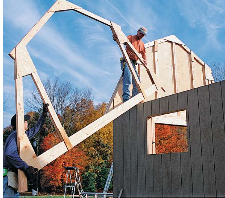
Greatly simplify the construction of a gambrel roof by building roof trusses on the ground. Then lift the trusses into place on top of the walls.
