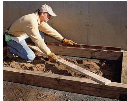
A timber-frame foundation rests on a compacted-gravel bed. Use a 4-ft. level to confirm that all four sides of the frame are perfectly level.
