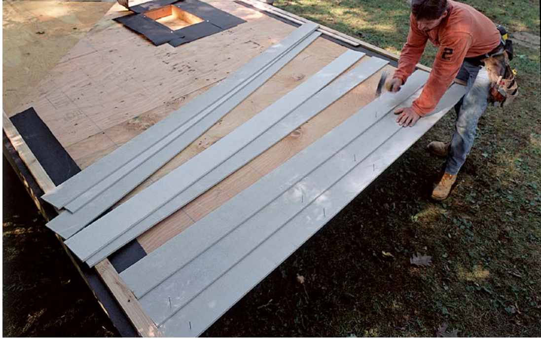
Cedar bevel siding , also called clapboards, is nailed to the walls in overlapping courses. The siding shown here comes preprimed and ready for paint.
