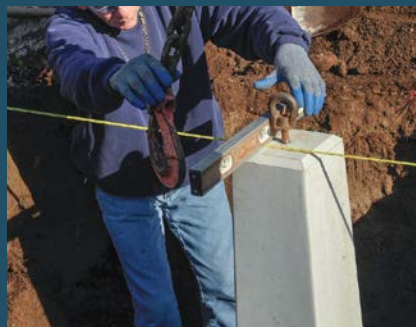
B. Confirm that the top of each concrete pier is level in two directions: front to back, and side to side. The piers must also be level with each other.
