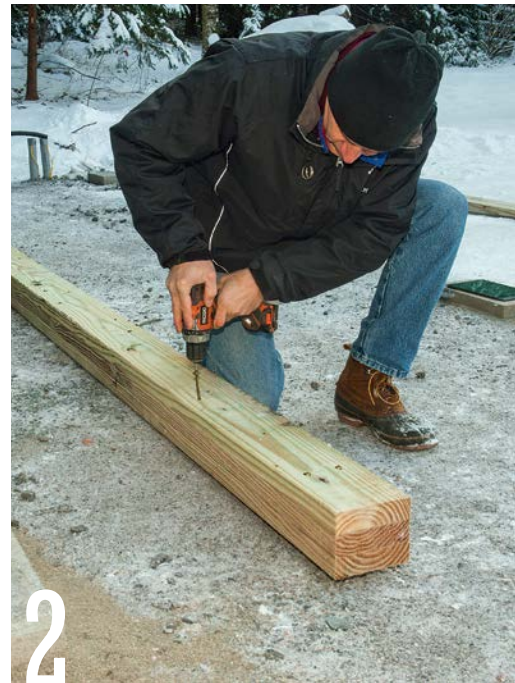
Make each 20-ft.-long skid by screwing together three pressure-treated 2×6s. Drive the 3-in. screws in from both sides of the skid.
