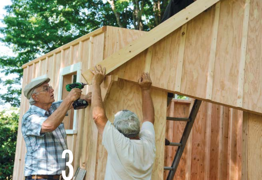
Raise one end of the truss about 2 ft., then move up the cleat. Repeat for the other end of the truss, slowly “walking” the truss up the wall.
