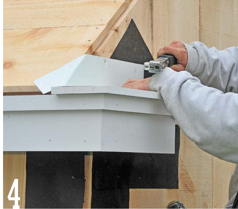
Staple a piece of aluminum flashing over the cornice-return cap. Be sure to staple only into the vertical flange, not into the horizontal cap.
