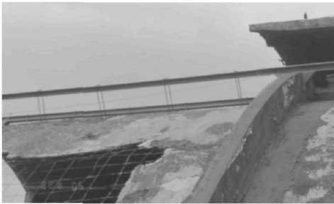
Figure 2 Partially collapsed shells
