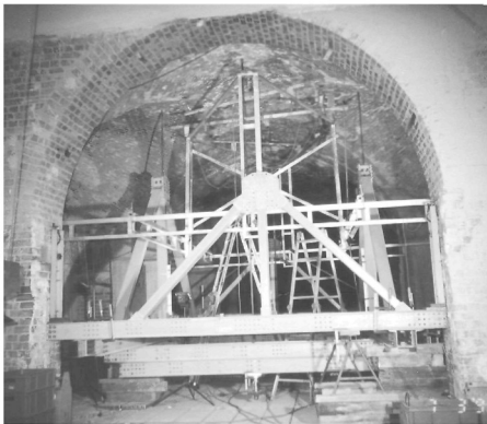
Figure 10 Loading and measuring device for a loading test on the arched vault damaged by fire
