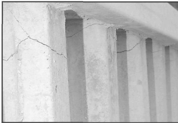
Figure 5 Typical failure of top end of posts (Tests 2 and 3)
