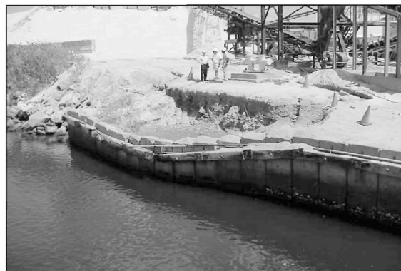
Figure 5 Concrete bulkhead dock wall impacted by a vessel
