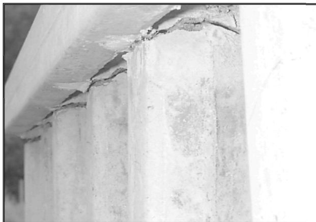
Figure 4 Typical bond failure between posts and handrail (Tests 1 and 4)
