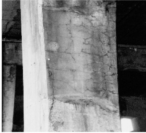
Figure 1 Corrosion around repair patch resulting from formation of incipient anodes
