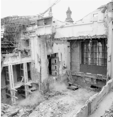
Figure 6 Cutting back the shear prestressed concrete walls with an oxygen lance and rope saw
