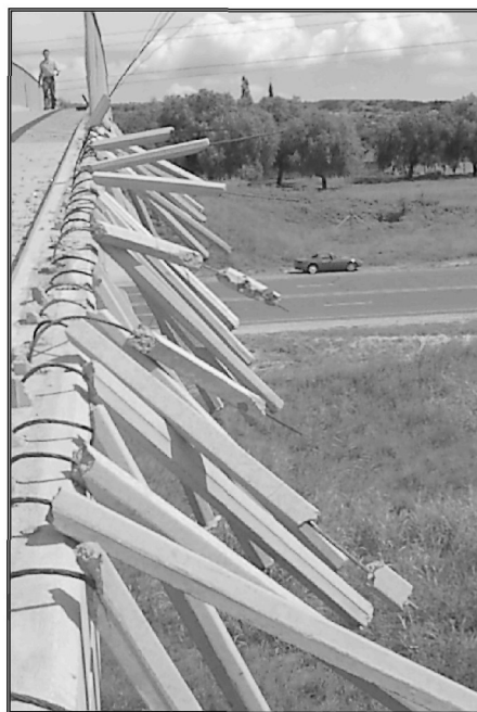
Figure 2 Damage to balustrades of Bridge B1831 over the N4
