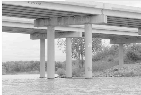
Figure 3 Two-column pier with ineffective collision wall at waterline due to high water conditions of waterway
